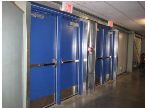
C4 exit doors leading to exterior from soccer fields on main level
