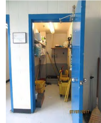
B33 Janitor's Closet (Upper Level): Space is too small to accommodate a universal washroom.
