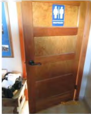
B13 Washroom #2 entrance. Washroom is not accessible. Generally, entrance doors are too narrow.
