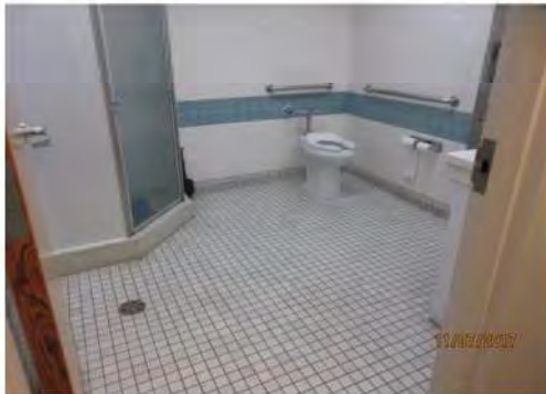
B40 1st floor, Unisex accessible washroom: Entrance clear width is suitable for existing condition. Interior floor space is suitable, including transfer space at side of toilet.
