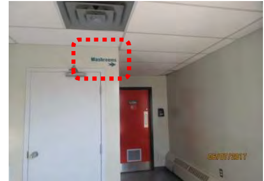
C3 Identification and directional signage for washrooms is not accessible and not highly visible (e.g., limited colour contrast and mounted too high).
