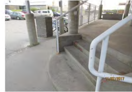
A18 Main Entrance: Stair handrail extensions are too short or not provided. No colour contrast is provided on stair nosings.
