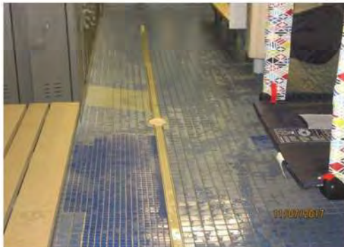
D16 Men's Change Room: Circulation clear width is typically limited for larger wheeled mobility aids. Cross-slope of some areas of floor surface is non-compliant and designed for drainage.
