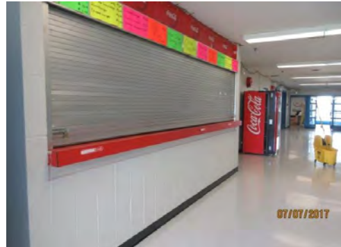
D2 Concession Stand (Upper Level): No lowered counter section is provided.
