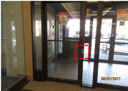
B4 Entrance (stair & ramp, 49th St.), interior side: A power door operator is provided, however, controls are too small. Accessible entrance is not marked with ISA decal.
