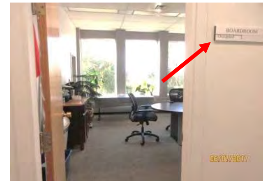
C12 Boardroom #213: Room identification signage does not have any accessibility features and is mounted too high.
