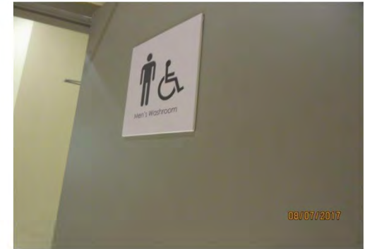
B57 Men's Accessible Washroom: Identification signage is not accessible, mounted on face of door. No braille / tactile features provided.
