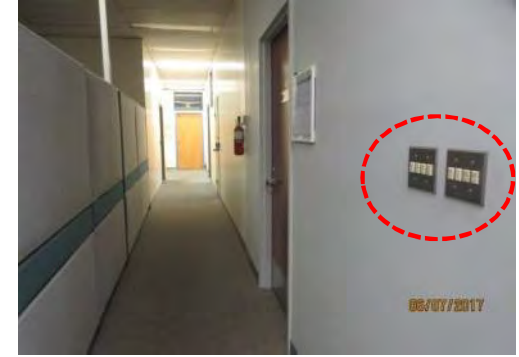
C3 Light switches (typical), 2nd floor corridor (sampled). Not mounted at accessible height.
