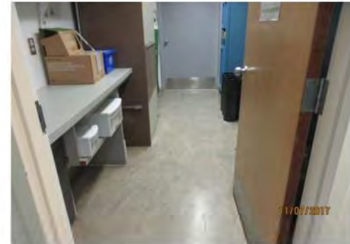
D3 1st floor, Equipment Room (off of central corridor): Clear door width is suitable for an existing condition. Knob door hardware is not accessible.
