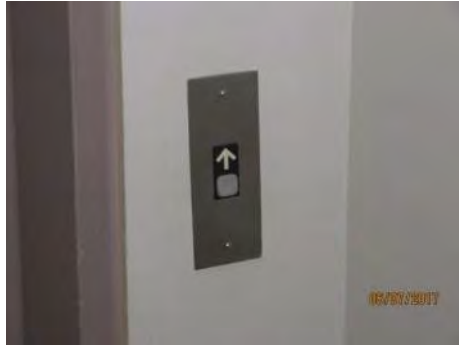
B50 Typical elevator hall call button. Arrow is raised and button illuminates when activated.
