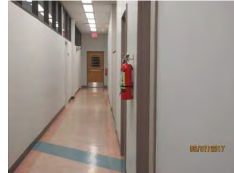
B33 2nd floor, Mayor's & Executive Offices, interior circulation: Generally, suitable clear width provided along central corridors. Base of fire extinguisher is not cane detectable for users with vision loss and extinguisher is a bumping hazard.
