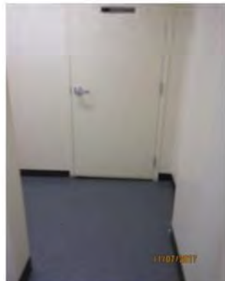
B30 1st floor, typical corridor, adjacent to Dormitory Entrance: Some floor space is limited with no clear turning space for users of mobility aids.
