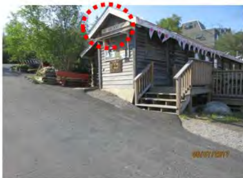
A10 Overhead building identification signage is mounted on façade but is generally not highly visible.
