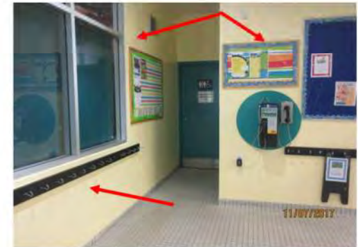
B18 Viewing Area: Coat hooks project into adjacent accessible route and approach to washrooms. Generally, information on display boards is posted too high.
