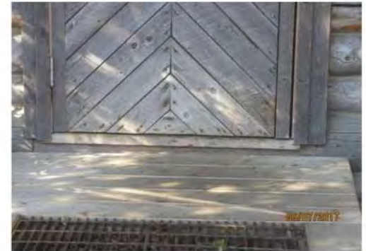
A9 Main entrance is not accessible due to elevation change and high threshold.
