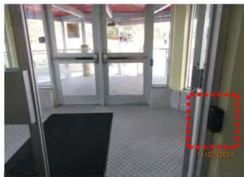
B5 Main entrance: PDO control is too small and mounted on door jamb.
