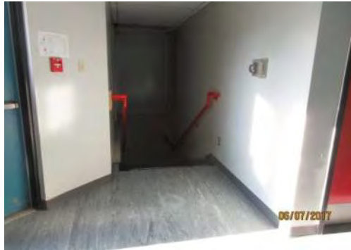
B25 View of approach to Stair #1 and secondary entrance / exit. No TWSI is provided at top landing.
