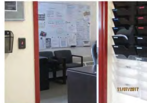
D6 1st floor, Dispatch / PSCC: Clear door width is suitable for an existing condition. Knob door hardware is not accessible. No accessibility features identified.
