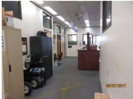
B43 2nd floor corridor (south side): Clear width and circulation is obstructed by temporary storage of items.
