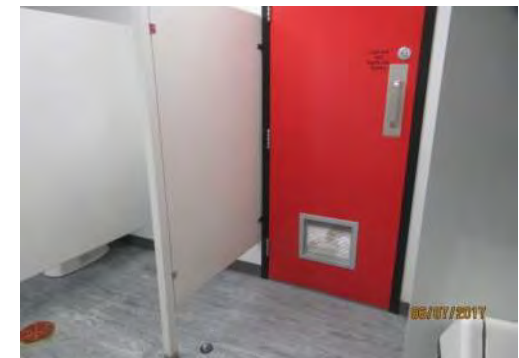
B48 Main Floor (adj. to secondary entrance): Men's Washroom. Identified as accessible through door signage but it is not accessible.
