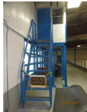
D11 Scorekeeper's Box, Upper Level: Open riser stairs are not accessible, however, it is recognized that this is a unique feature with no public access.
