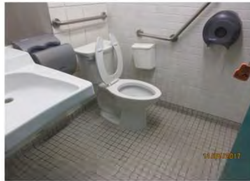
B20 Unisex washroom: Not identified as accessible through door mounted signage. Interior floor space is very limited. Grab bars are provided at toilet.
