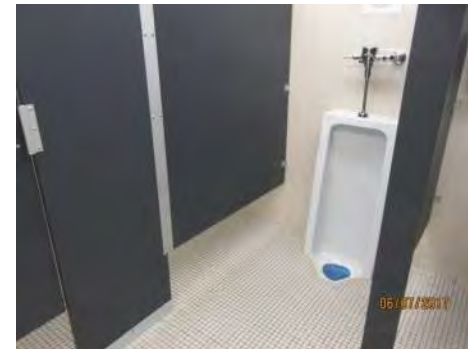
B90 Men's Accessible Washroom, main floor: A lowered, floor mounted urinal is provided, however, flush control is mounted too high.
