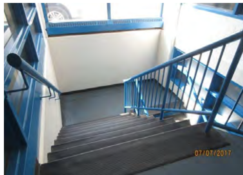
B16 Central Stair: No colour contrasted nosings provided. Handrail grasping dimension is too large. No handrail extensions are provided at top landing.
