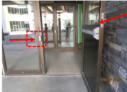
B14 Entrance (Sloped route), exterior vestibule door: Lower edge of glazing is too high. Clear width is suitable for existing. Exterior door is not marked with ISA decal.
