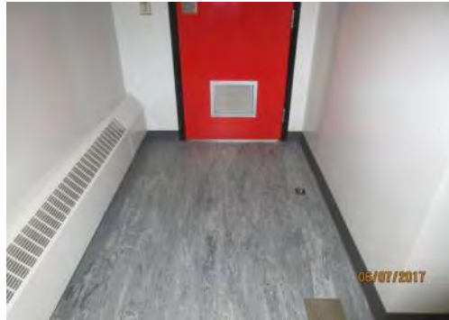
B43 Main Floor (adj. to secondary entrance): Women's Washroom. Identified as accessible through door signage but it is not accessible.
