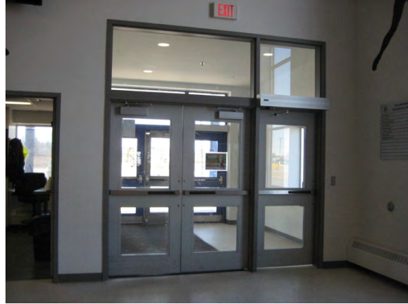
B2 Vestibule doors – note power operator for single door to right
