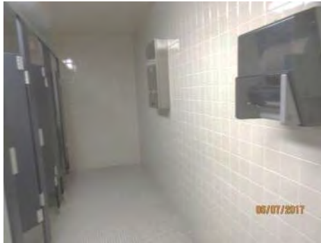
B115 2nd Floor, Women's Accessible Washroom (Staff): Limited clear floor space in front of entry to accessible stall. Accessible stall dimensions are limited.
