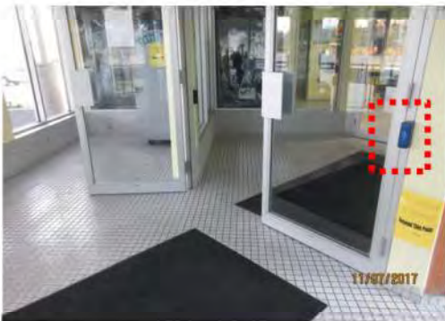
B4 Middle door, between vestibule & foyer: Suitable clear width is provided. PDO control is small (typical) and mounted on door jamb (typical).
