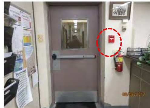
C11 Exit, main floor (south east side): Typical fire pull stations are mounted too high.
