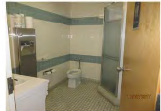
B42 1st floor, Unisex washroom: Not identified as accessible through door signage. Knob door hardware is not accessible.
