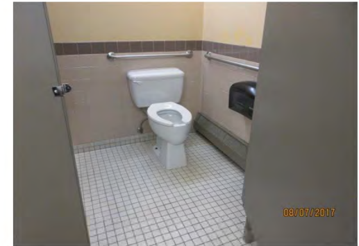
B75 Women's Accessible Washroom: Stall has limited clear floor space. Door clear width is too narrow.
