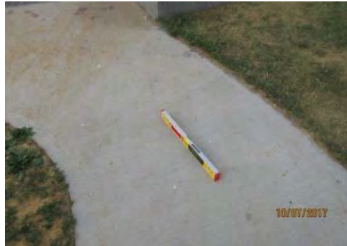
D66 Somba K'e Service Building (exterior): Walkway is narrow. Running slope of walkway to entrance is too steep in multiple sections, for users of mobility aids, exceeding 11%.
