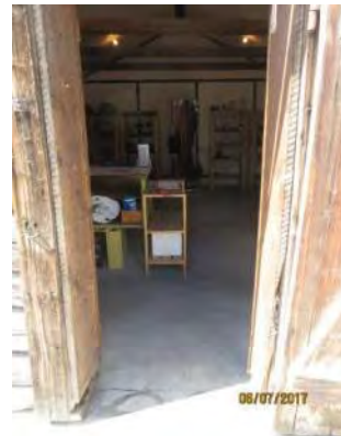
D107 Fireweed Studio (exterior): Level transition at entrance. Clear door width is too narrow
