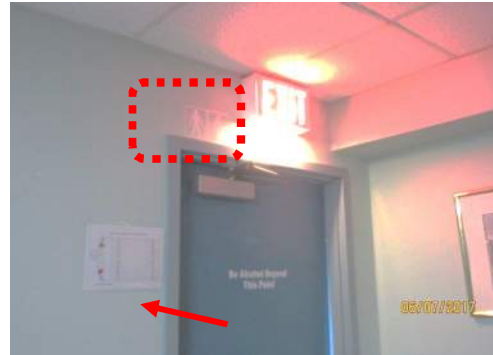
C2 Fire safety plans are provided adjacent to exits. Identification and directional signage for washrooms is not accessible and not highly visible (e.g., limited colour contrast and mounted too high).
