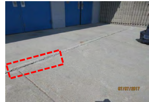
A9 Approach to main entrance (west side). Some heaving / settlement between concrete sections observed.
