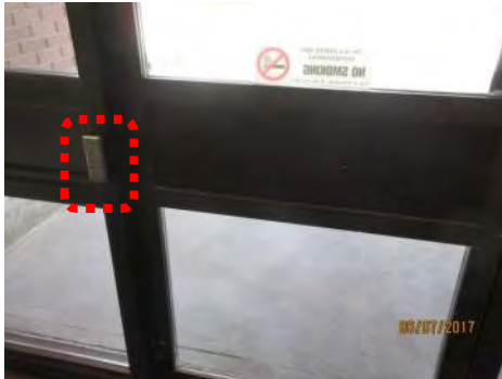
B5 Accessible entrance (south side): Power door operator control (interior) is too small and difficult to locate.
