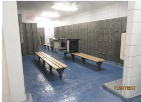
D14 Men's Change Room: Typical bench seating is too low. No accessible lockers identified through signage and/or operating hardware
