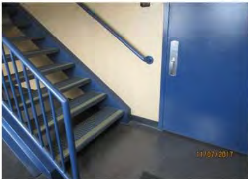
B18 Central staircase: No handrail extensions provided (typical). Limited clear floor space at bottom landing and adjacent to entrance door to 1st floor.
