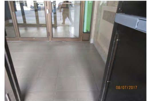
B15 Entrance (Sloped route): View of interior vestibule. Limited clear floor space between doors when interior vestibule door is open at 90 degrees.
