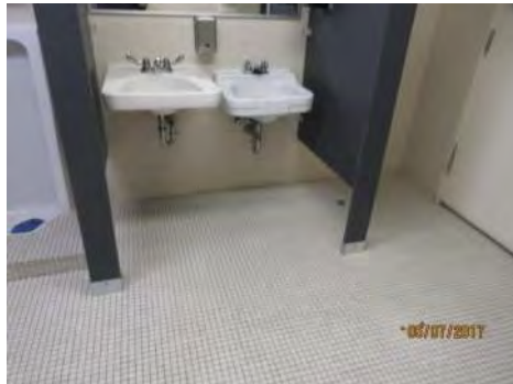
B109 2nd Floor, Men's Accessible Washroom (Staff): Lavatory configuration and mounting is non-compliant.
