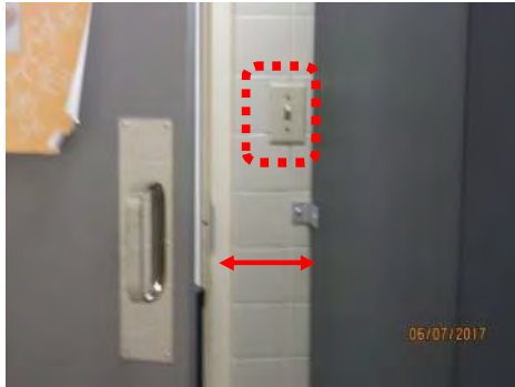
B97 Women's Accessible Washroom, main floor: Light switch is mounted too high.
