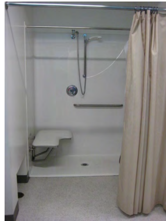
D20 shower stall in upper level change room (typical)
