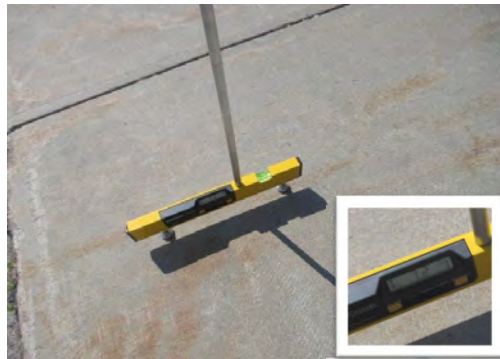
A13 Concrete surface, adjacent to main entrance: Excessive cross-slope at 7.2%.
