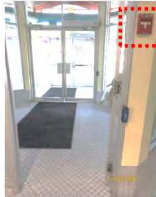
C2 Entrance Foyer, Fire pull is mounted too high, at 1500 mm +.
