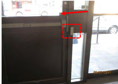
B7 Entrance (stair & ramp, 49th St.): Exterior door glazing is mounted too high. Power door operator control is too small.
