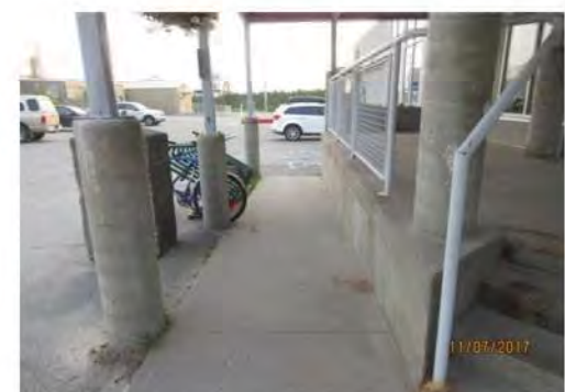
A12 View of approach to and from main entrance. Surface of accessible route is in good condition.
