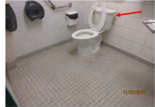
B21 Unisex accessible washroom: Generally, interior floor space is non-compliant and limited clear turning circle (less than 1500 mm), as well as interior amenities. Manual flush control is not on transfer side of toilet. Transfer space at side of toilet is too small.
