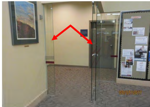
B55 Entry vestibule (washroom area): Clear door width is too narrow and non-compliant. Edges of glazing are not clearing marked for users with vision loss, resulting in potential bumping hazards.
