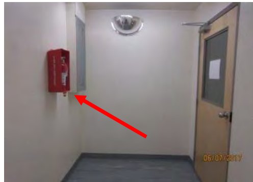
C5 Fire extinguisher cabinet projects from wall, with no cane detection feature at base for users with vision loss.
