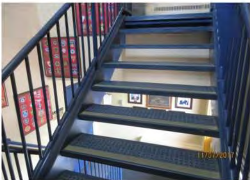
B17 Central staircase: Open risers are not accessible. Colour contrasted & slip-resistant stair nosings are provided.
