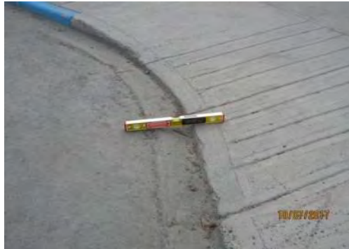
A7 Curb ramp (south east side, adj. to on-street accessible parking space): Transition between roadway and curb ramp surfaces is too high.
