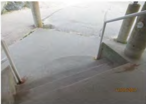
A19 Main Entrance: No colour contrast is provided on stair tread nosings. No tactile warning surface indicator is provided at top of stair landing.
