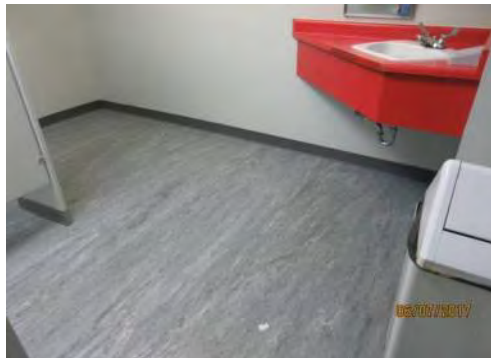
B35 Main Floor (adj. to entrance): Men's Washroom. Identified as accessible through door signage but it is not accessible.
