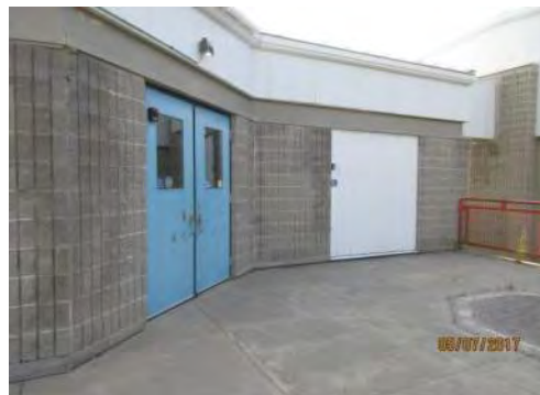
A11 Main entrance: Level access is provided for users of mobility aids. Entrance is not marked as accessible through signage.
