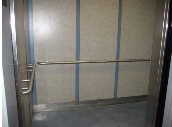
B19a Elevator car interior
