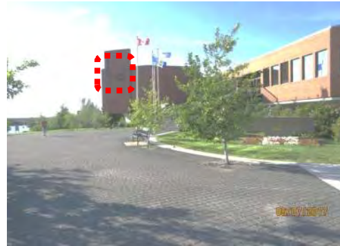
A2 Colour / tonal contrast is limited for exterior signage (mounted on façade).
