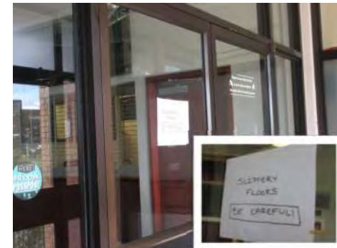
B18 Main entrance (west side): Temporary signage is posted to advise that floors are "slippery".
