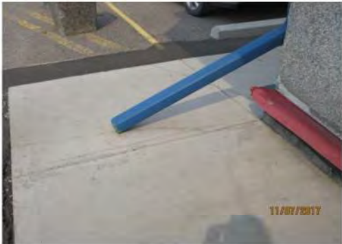
A20 Main entrance area: Eave trough obstructs clear width and is a potential tripping hazard.
