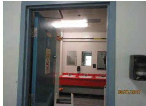
D35 Women's Changeroom (Lower Level): Entrance door clear width is too narrow.
