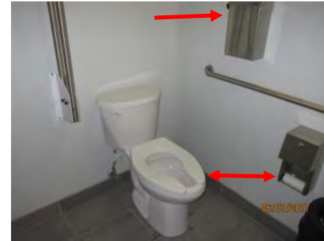
B105 2nd Floor, Universal Washroom: Toilet paper dispenser is mounted too far from front edge of toilet. Sanitary dispenser is mounted too high on side wall. Flip-down grab bar requires adjustment.
