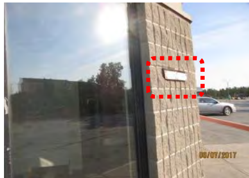
C4 Exterior entrance identification sign is worn / faded, with no accessibility features (e.g., large text / colour contrast etc.).
