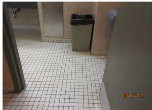
B71 Women's Accessible Washroom: Limited interior clear floor space, especially for users of larger wheeled mobility aids.
