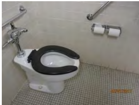
B100 Women's Accessible Washroom, main floor: Interior features / floor space are non-compliant, including accessible stall dimensions.
