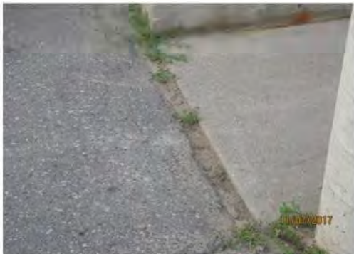
A10 View of approach to and from main entrance, adjacent to accessible parking spaces. Some minor disrepair between concrete and asphalt surfaces. Approach to accessible route can potentially be obstructed when vehicle is parked in space.
