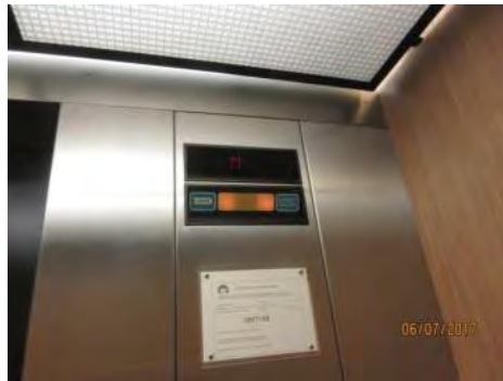
B52 Elevator: LED visual indicator (floor level).
