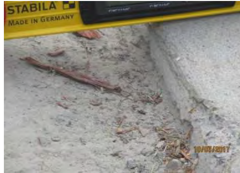
A8 Curb ramp (south east side, adj. to on-street accessible parking space): Transition between roadway and curb ramp surfaces is too high.
