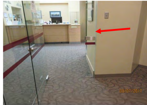
B56 Entry vestibule (washroom area): Edges of glazing are not clearing marked for users with vision loss, resulting in potential bumping hazards.
