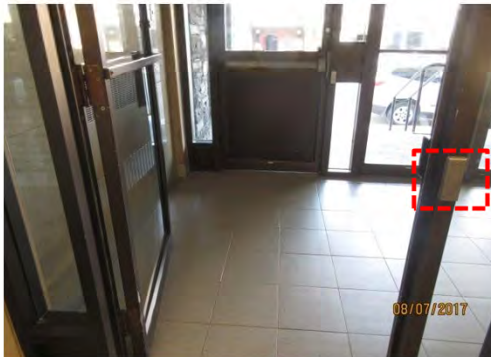
B5 Entrance (stair & ramp, 49th St.), interior side: Suitable clear width is provided. Power door operator control is too small and ISA symbol has faded.
