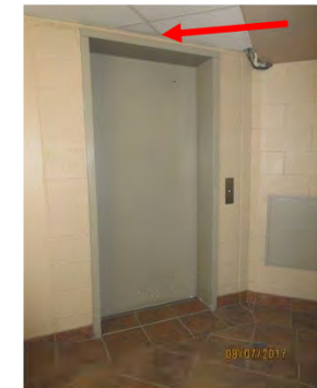
B51 Elevator lobby, parking garage. No overhead or side panel visual indicator is provided.
