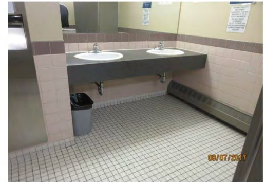
B63 Men's Accessible Washroom: No accessible lavatory with required knee space below is provided.
