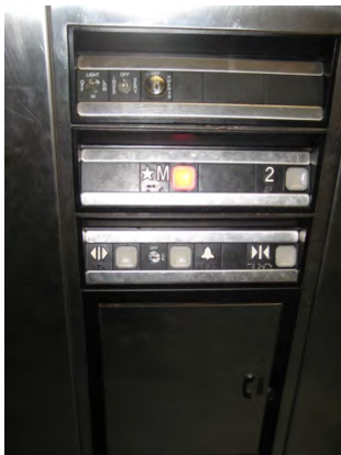
B19b Elevator controls
