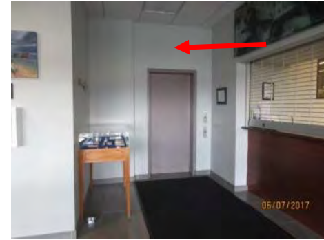
B57 No overhead elevator cab position (visual indicator) is provided.
