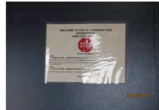
C6 Main entrance vestibule: Information and instructional signage is mounted too high with no accessibility features.
