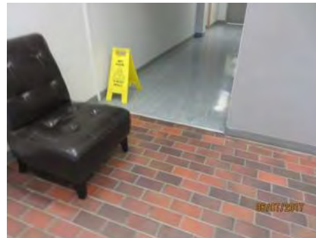
B11 South entrance, main floor: Chair obstructs clear width of accessible route and corridor to elevator.
