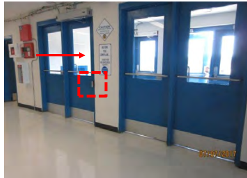
B8 View of main entrance and vestibule from interior side: Accessible door and power door operator control is not marked with ISA decal.
