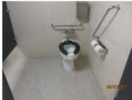
B116 2nd Floor, Women's Accessible Washroom (Staff): Interior features / floor space are non-compliant, including accessible stall dimensions and grab bars.
