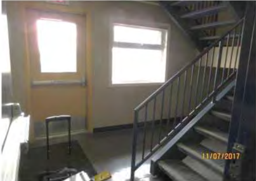
B20 Central staircase: Limited clear floor space adjacent to main entrance door.
