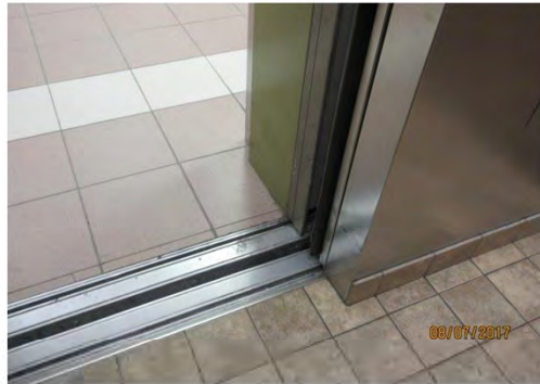
B43 Elevator: Suitable clear width is provided at entry, however, door closes too quickly.
