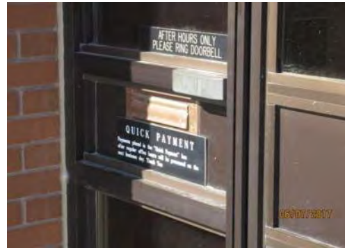
C14 Exterior signage is dated, with inconsistent design and features.
