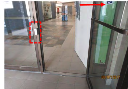
B18 Entrance (Sloped route), interior vestibule door: Level access is provided. Clear width and threshold is suitable. Interior door only is marked with ISA. Power door operator control is small.
