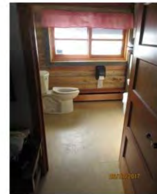
B12 Washroom #2: Washroom is not accessible. Limited interior clear floor space. Entrance doors are too narrow.
