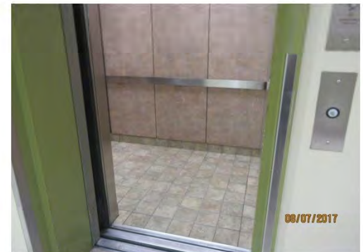
B42 Elevator: Generally, interior floor space is compliant, however, features require modernization.
