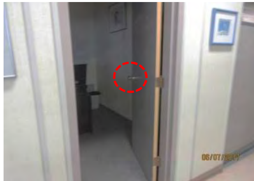
D46 Private Office, 2nd floor (east side). Typical entrances have limited clear width and knob door hardware which is not accessible.
