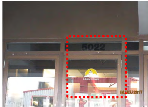
A20 Library entrance is marked with door identification signage, however, it is difficult to identify from a distance.
