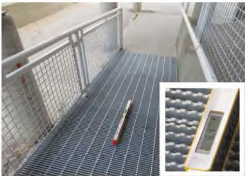
A26 Ramp: Running slope is technically non-compliant and too steep at 8.4%, however, it is assumed grating can potentially be adjusted.
