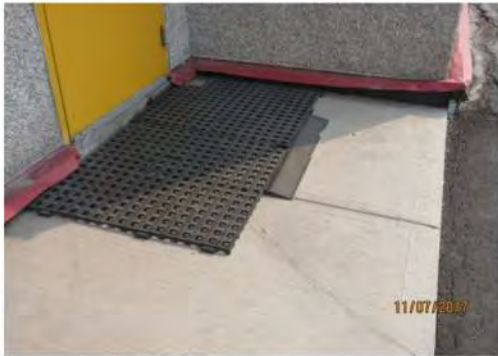
A15 Main Entrance: Stepped access only. Ramped threshold is in disrepair.
