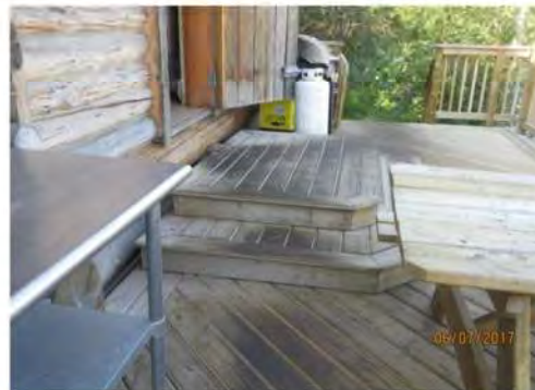
A17 Secondary entrance (side): Stepped access only.
