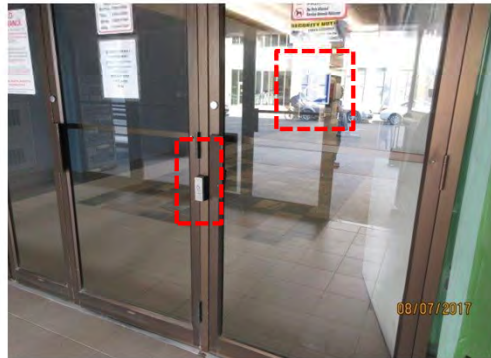
B17 Entrance (Sloped route), interior vestibule door: Door is marked with ISA decal. Power door operator control is small. Adjacent door swings toward user and power door operator control and is potential bumping hazard.
