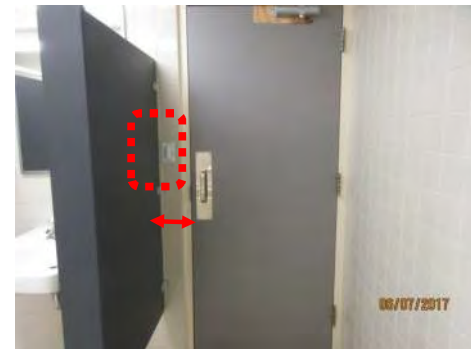
B93 Men's Accessible Washroom, main floor: Interior features are non-compliant. Occupancy light sensor is provided. Clear wall space at latch side of door for approach to & use of door hardware is not provided.
