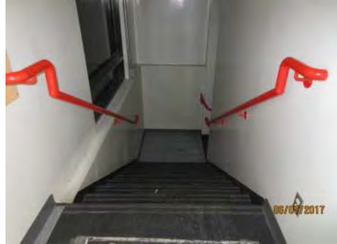
B26 Stair #1: No colour contrast is provided on stair tread nosings for users with a vision loss. Handrails have large grasping surface / dimension.
