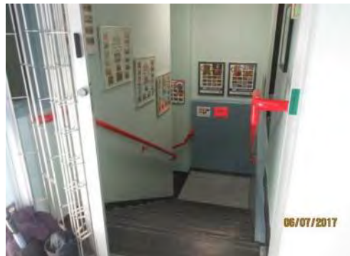
B29 Stair #2: No colour contrast is provided on stair tread nosings for users with a vision loss.
