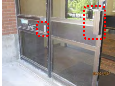
B2 Accessible entrance (south side): Power door operator control (exterior) is too small and difficult to locate. Door hardware is not accessible.
