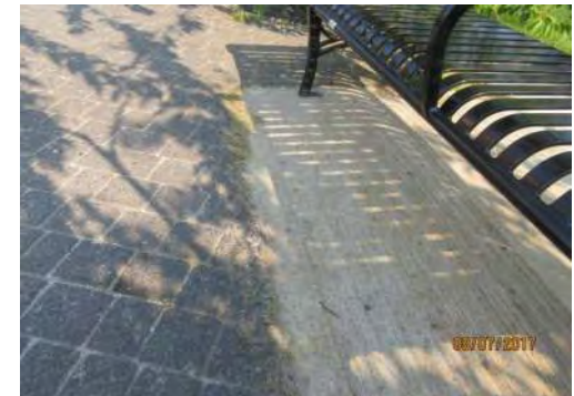
A36 Transition between edge of concrete and brick paver surfaces is uneven and sloped, which results in potential tripping hazard.
