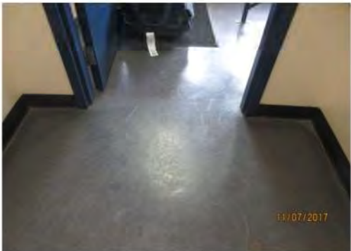
B22 1st floor, entrance vestibule (interior door): Clear width is too narrow but suitable for existing condition. Main entrance is not accessible for users of mobility aids.
