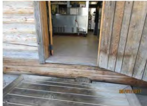
B2 View of entrance at side, off of exterior deck, with stepped entry only.
