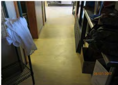
B16 Staff work area. Corridor to kitchen and exterior patio. Clear width is not accessible for users of mobility aids.
