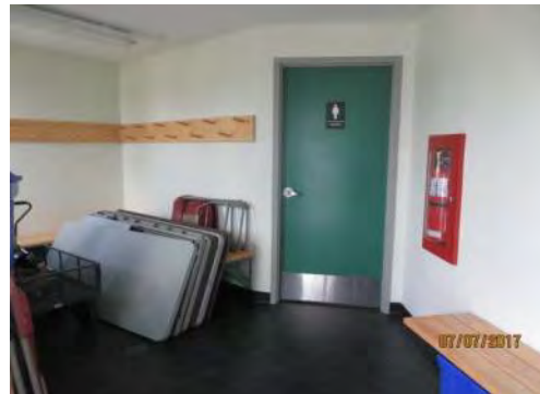
D89 Somba K'e Service Building (interior): Washrooms are not identified as accessible through door mounted signage. Signage is not accessible.
