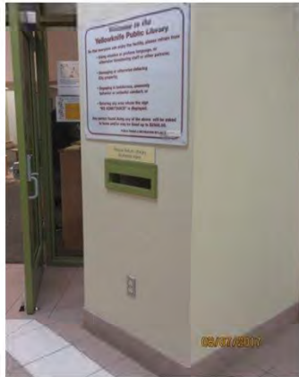
C19 Book Return and Information Signage: Suitable colour contrast is provided. Print size is typically small, with no braille / tactile features or alternate accessible signage provided.
