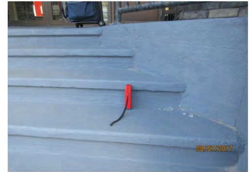
A21 Stairs: No colour contrasted nosings are provided. A centre handrail is provided only. No handrails are provided on other sides of stairs.
