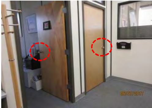
D55 Staff work area, 2nd floor (south side): Typical private offices. Typical knob door hardware is not accessible.
