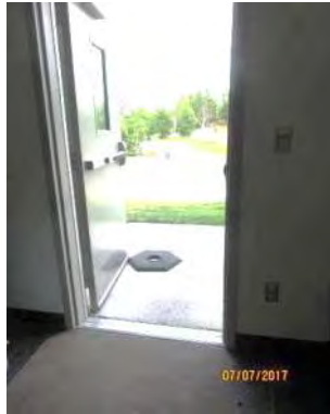
D85 Somba K'e Service Building (interior): Main entrance is not accessible with limited clear width and high glazing.
