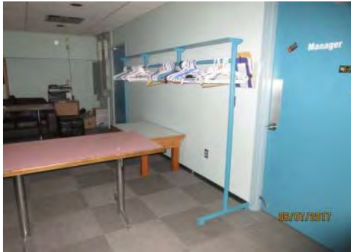
D1 Manager's Office (upper level): Door clear width and knob door hardware is not accessible.
