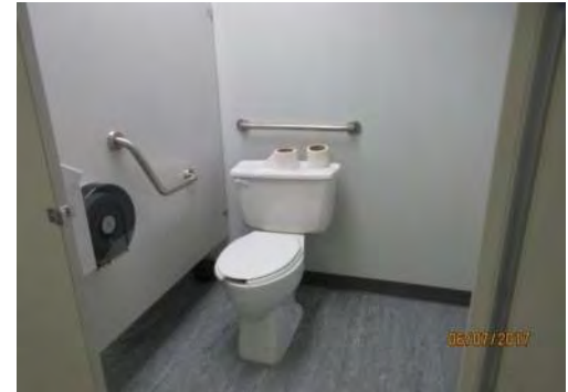
B39 Women's Washroom (adj. to entrance): Identified as accessible through door signage but it is not accessible. Stall dimensions non-compliant.
