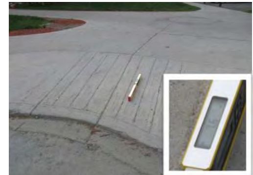
A6 Curb ramp (south east side, adj. to on-street accessible parking space): Running slope is suitable at 7.6 percent. No TWSI is provided. Transition between roadway and curb ramp surfaces is too high.
