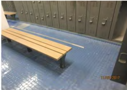
D13 Men's Change Room: Circulation for users of mobility aids is limited. Typical bench seating is too low. No accessible lockers identified through signage and/or operating hardware, however, some lower lockers may be adaptable.
