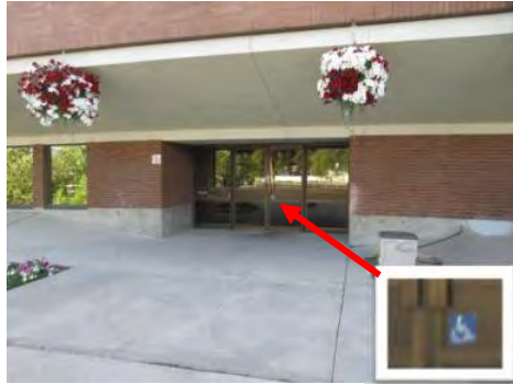
B1 Approach to accessible entrance (south side). Exterior accessible door is marked with International Symbol of Accessibility, but interior doors are not.
