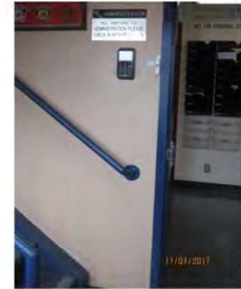
C3 Main entrance lobby, directional signage and security pad: Generally, no accessibility features identified.
