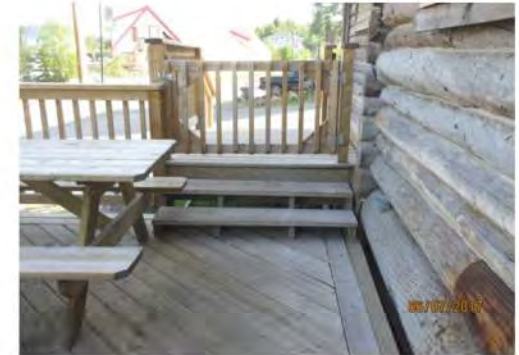
A15 Stepped access only is provided to exterior deck. No colour contrasted nosings are provided. Handrail is oversized. Open risers are not accessible.
