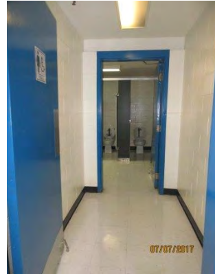
B20 Women's Accessible Washroom (Upper Level): Entrance doors have limited clear width but suitable for an existing condition. Door mounted signage is not accessible. No power door operators are provided.
