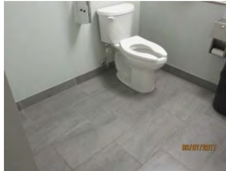
B104 2nd Floor, Universal Washroom: No clear turning circle due to wall at entrance vestibule.
