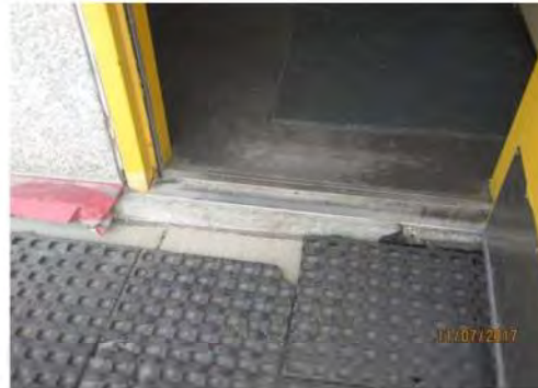
B2 Main entrance (north side): Stepped entry only, due to high threshold. Entrance is not accessible.
