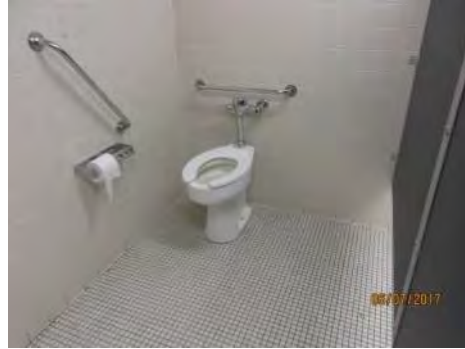
B92 Men's Accessible Washroom, main floor: Interior features are non-compliant.
