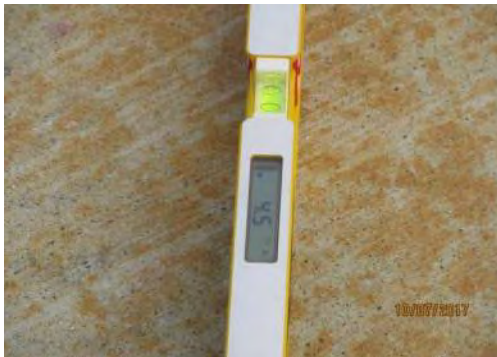
D75 Somba K'e Service Building (exterior): Running slope of walkway to entrance (lower section) is suitable in some areas, for users of mobility aids, at 5% or less.
