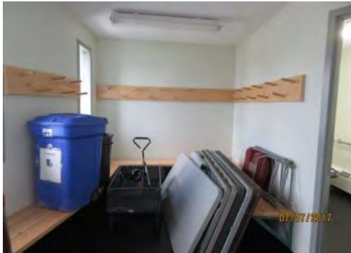
D91 Somba K'e Service Building (interior): Many interior areas are used for storage. Clear floor space is limited. Clothes hooks are mounted too high.
