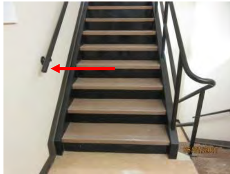
B79 Stair #1 (northeast side): No handrail extensions are provided at bottom landings. No colour contrasted nosings on stair treads.
