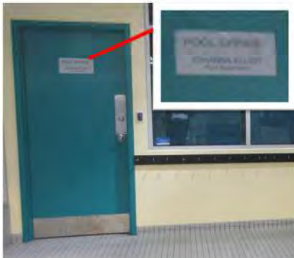
C4 Generally, space identification signage is dated and/or temporary, with no accessibility features provided (e.g., braille / tactile).
