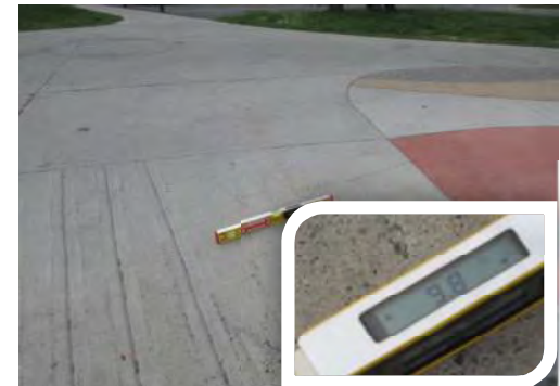
A9 Curb ramp (south east side, adj. to on-street accessible parking space): Running slope of flared side is suitable at 9.8%.
