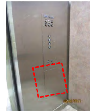
B45 Elevator cab control panel: No braille / tactile signage provided. No emergency phone appears to be provided with no handle on cabinet door. No emergency phone is identified through signage.
