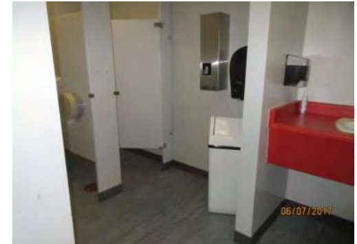
B45 Main Floor (adj. to secondary entrance): Women's Washroom. Identified as accessible through door signage but it is not accessible.
