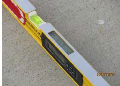
D67 Somba K'e Service Building (exterior): Walkway is narrow. Running slope of walkway to entrance is too steep for users of mobility aids, exceeding 11%.
