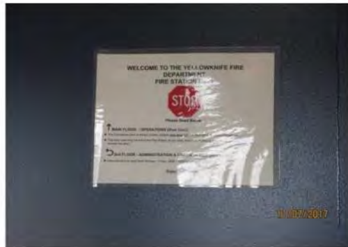
B7 Main entrance vestibule: Information and instructional signage is mounted too high with no accessibility features.
