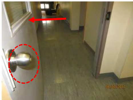
B58 Entrance, main floor (adj. to corridor to elevator lobby): Knob door hardware is not accessible. Lower edge of glazing is mounted too high.
