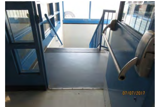
B15 Entrance to Central Stair: Thumb-latch door hardware is not accessible. Lower edge of glazing is too high but there is additional glazing as part of sidelights that enhances visibility to prevent any potential bumping hazards.
