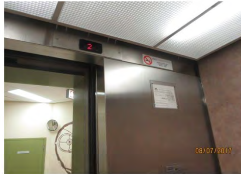
B44 Elevator: Overhead LED panel is provided inside cab to indicate floor level.
