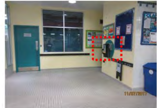
C3 Some telephone controls are mounted too high, above 1200 mm from floor. Lower edge is not cane detectable for users with vision loss when approaching from sides. No overhead signage is provided at corridor to washrooms to assist with their identification.
