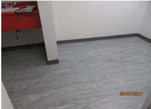
B49 Main Floor (adj. to secondary entrance): Men's Washroom. Identified as accessible through door signage but it is not accessible.
