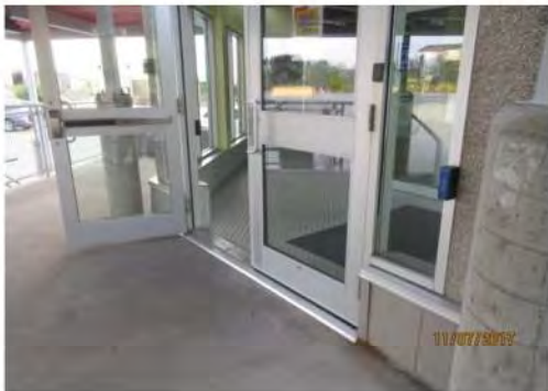
A21 Main entrance: One door leaf is equipped with power door operator. Accessible door is not marked with International Symbol of Accessibility decal. Power door operator control is too small and difficult to identify.
