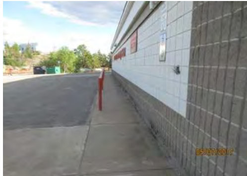
A7 Approach to secondary entrance: Clear width of sidewalk is reduced significantly by guardrail.
