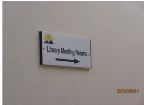
C11 Meeting Room: Directional signage text is too small.
