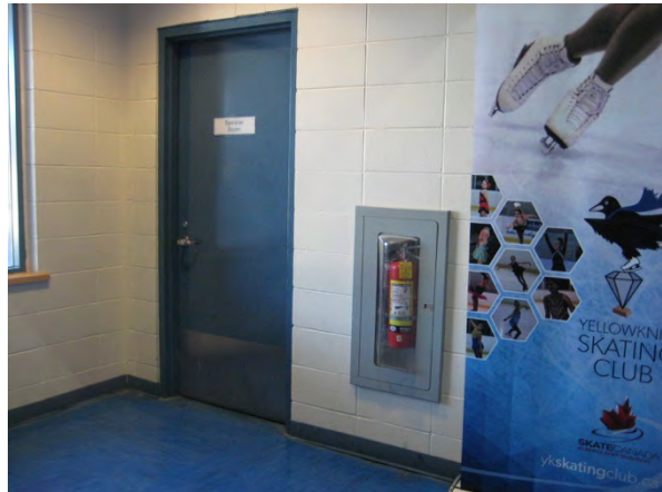
C10 ID Fire extinguisher cabinet (typical)
