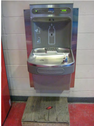
C13 water fill station lobby main floor
