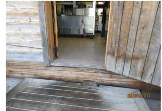
A21 Secondary entrance (side): Stepped access only.
