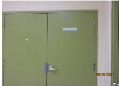
D2 Entrance to Meeting Room: Identification signage text is too small with limited colour contrast. Lever door hardware is accessible. Clear door width is suitable if double doors activated at same time.
