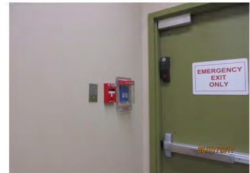
C18 Exit Stair (adj. to Meeting Room): Fire alarm pull is mounted too high. Appeared to be typical condition throughout.
