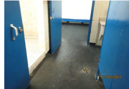
D33 Shared Shower / Washroom, Change Rooms #3 & #4 (Lower Level, north side): Limited interior floor space for shared facilities.
