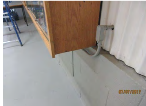
D8 Corridor & Viewing Area (Upper Level, south side): Cabinet projects with no cane detectable bottom edge for users with vision loss.
