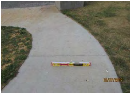
D72 Somba K'e Service Building (exterior): At lower section of walkway, cross-slope is suitable at 2% or less. Walkway is narrow.
