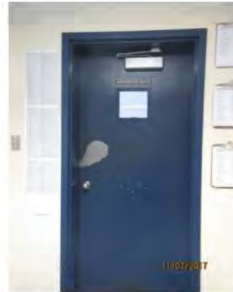
C2 1st floor, typical door mounted signage, Entrance to Apparatus / Truck Bays: Interior signage is limited, with no accessibility features.
