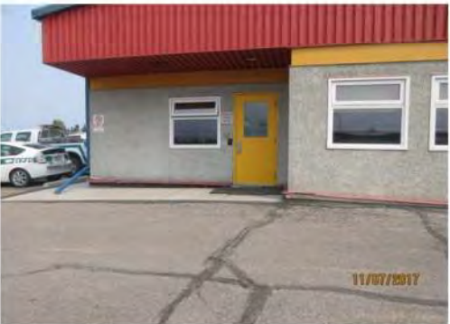
A12 Main entrance: No accessibility features identified.
