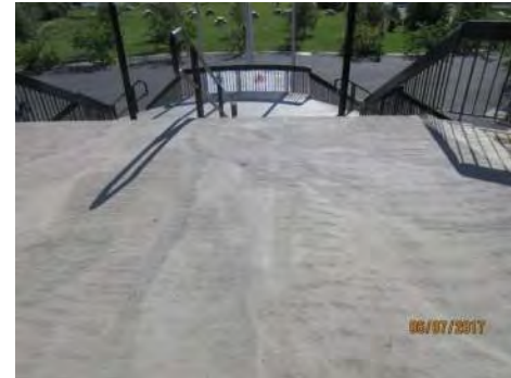
B12 West entrance is not accessible for users of mobility aids due to stair access only.
