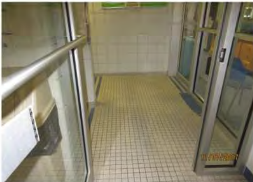
B16 Entry vestibule to Change Rooms & Staff Areas (exterior side): Clear door width is limited.
