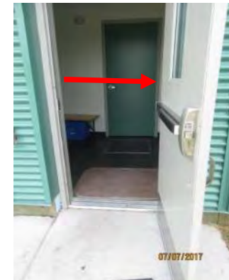
D84 Somba K'e Service Building (exterior): Main entrance is not accessible with limited clear width and high glazing. Push bar hardware reduces clear width.
