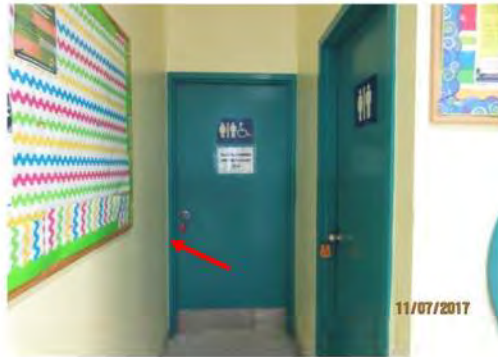
B19 Corridor and approach to washrooms. Limited clear width provided throughout corridor. No wall clearance at latch side of door is provided (Red arrow). No power door operator is provided.
