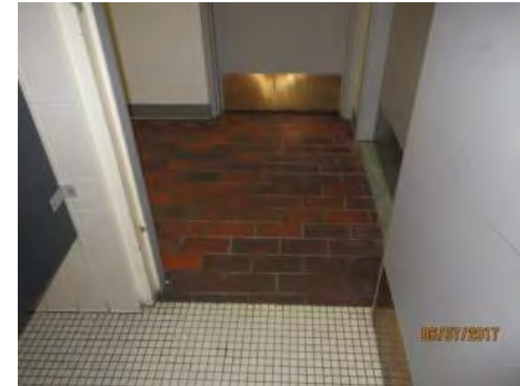
B87 Men's Accessible Washroom, main floor: Identified as accessible through door signage. Clear door width and interior features are typically non-compliant.
