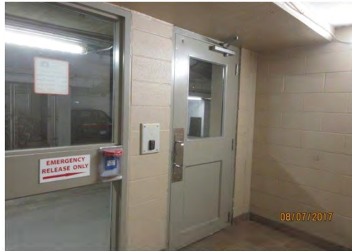
B49 Elevator lobby, parking garage. Door was secured at time of audit. No power door operator is provided.
