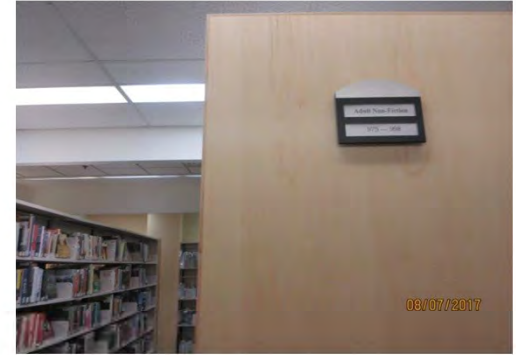
C3 Typical stack signage, (Adult-non-fiction 973-998): Colour contrast is suitable, however, mounting is too high and print size is small for legibility. No braille / tactile features or alternate accessible signage provided.
