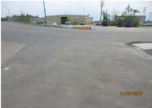
A8 Taylor Road, intersection of public sidewalk and driveway to parking lot: Drive aisle is not marked. no linked, accessible route to main entrance.
