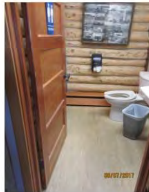
B11 Washroom #1 entrance. Washroom is not accessible. Limited interior clear floor space.
