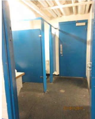
D49 Shared Shower / Washroom, Change Rooms #1 & #2 (Lower Level, south side): Limited interior floor space for shared facilities.
