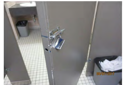
B66 Men's Accessible Washroom: Stall door hardware is not accessible.
