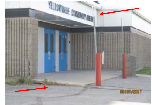
A6 View of facility identification signage and main entrance to Arena. A high transition was identified at one side, with no curb ramp and no direct and linked accessible route that could lead to adjacent Curling Club.
