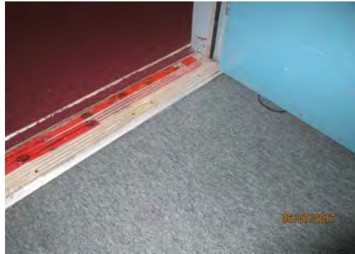
D13 Curling Rink (accessed from Lower Level): Level access at entry #2 and suitable clear door width is provided for an existing condition, however, no elevator access is provided to this level.
