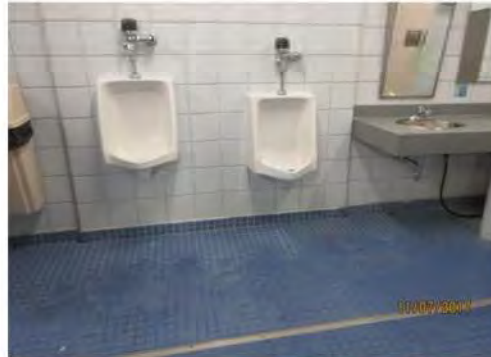
D17 Men's Change Room: A lowered urinal with auto flush control is provided. No upgrade is recommended for this feature since facility is scheduled for replacement.
