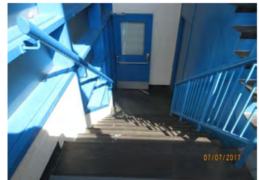
B18 Central Stair: No colour contrasted nosings provided. Handrail grasping dimension is too large. No handrail extensions are provided at intermediate landing.
