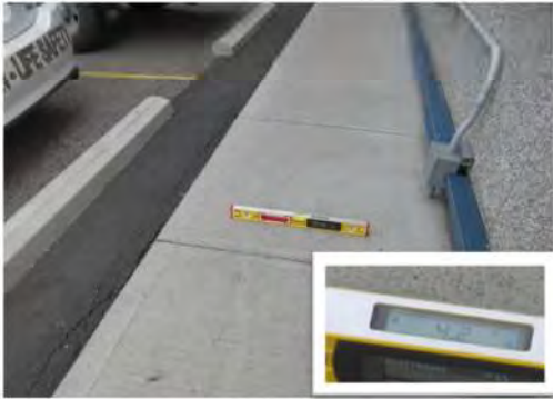
A23 Approach to staff entrance / exit (east side): Cross-slope too steep at 4.2%.
