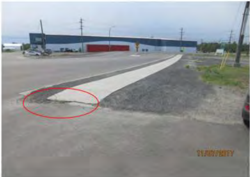
A7 Taylor Road, public sidewalk, west side of site. No compliant curb ramp and no linked, accessible route to main entrance. No tactile warning surface indicator is provided. No site signage and / or parking lot identification signage.
