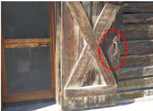
D106 Fireweed Studio (exterior): Clear door width is too narrow. D-pull hardware is small size with limited colour contrast.
