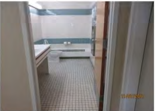
B35 2nd floor, entrance to Washroom #2: Clear width is suitable. No accessibility features identified. However, 2nd floor is not accessible.
