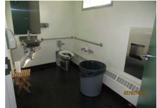
D93 Somba K'e Service Building (interior): Women's washroom is not accessible although some accessibility features are provided (e.g., grab bars). No transfer space is provided at side of toilet. Interior floor space is limited.
