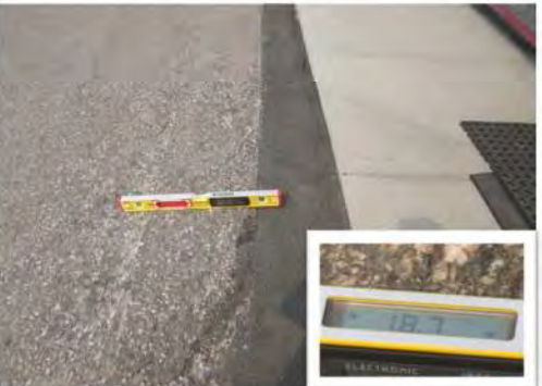
A17 Considerable slope of 18.7%, at transition between drive aisle and sidewalk at main entrance, when approaching for parking lot.
