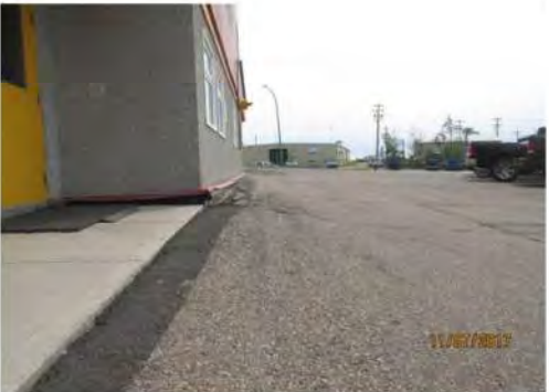
A16 Main entrance area: Considerable slope at transition between sidewalk and drive aisle.
