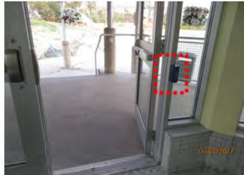
B2 Exterior door: Suitable clear width is provided. PDO control is small (typical) and mounted on door jamb (typical).
