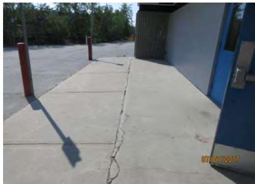
A10 Approach to main entrance (looking towards south side of site). Some heaving / settlement between concrete sections observed. Excessive cross-slope in some areas, exceeding 2%.
