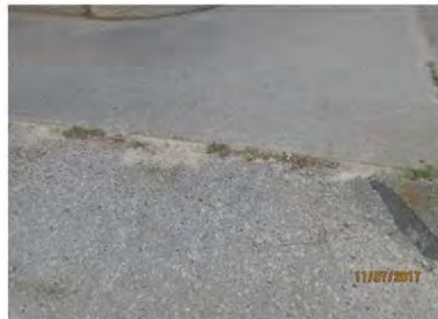
A17 Approach to Main Entrance: Some settlement & heaving between concrete & asphalt surfaces, resulting in potential tripping hazard.
