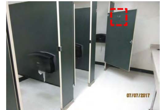
B30 Men's Accessible Washroom (Upper Level): Stall doors are not self closing. Coat hook is mounted too high.
