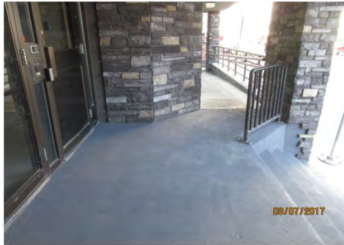
B1 Entrance (stair & ramp, 49th St.): Accessible entrance is not marked with ISA decal. Top landing of ramp is awkward configuration.
