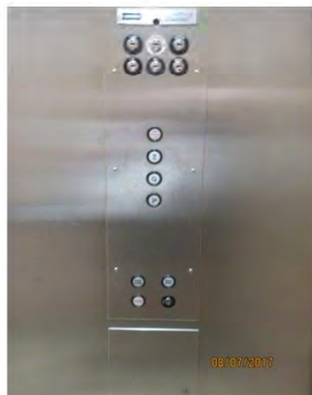
B46 Elevator cab control panel: No braille / tactile signage provided. Some buttons are mounted too high for users of wheeled mobility aids.
