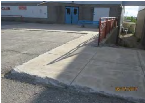
A13 No curb ramp is provided. No informational or directional signage is provided to guide users to main entrance.
