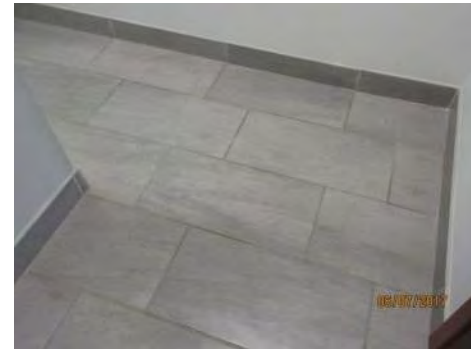
B102 2nd Floor, Universal Washroom: Entrance vestibule is too narrow (clear width), especially for larger wheeled mobility aids.
