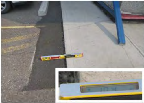
A21 Main entrance area: Considerable slope at transition between sidewalk and drive aisle at 10.4%.
