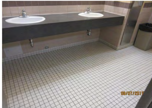
B73 Women's Accessible Washroom: No accessible lavatory with required knee space below is provided.
