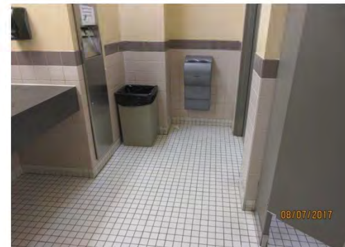
B72 Women's Accessible Washroom: Limited interior clear floor space, especially for users of larger wheeled mobility aids.
