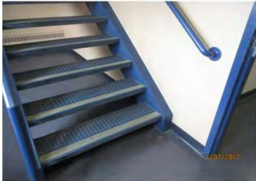
B19 Central staircase: Limited clear floor space at bottom landing and adjacent to entrance door to 1st floor.
