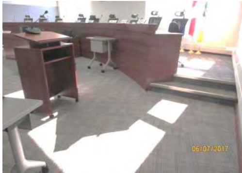
D13 Council Chamber: Speaker's Podium. No accessibility features identified.
