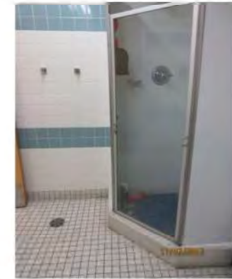
B39 1st floor, Unisex accessible washroom: Shower is not accessible due to stepped / curbed entry.
