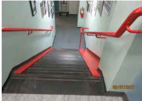
B31 Stair #2: Handrails have large grasping surface / dimension. No colour contrast is provided on stair tread nosings for users with a vision loss.
