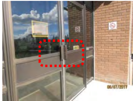
B14 Main entrance (west side): Door hardware is not accessible for users with limited manual dexterity.
