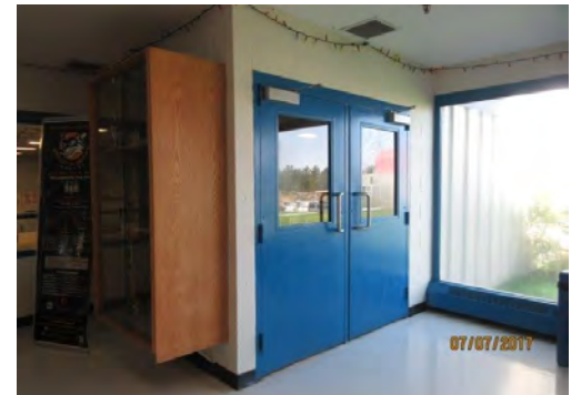
B9 Entrance to seating stands and Ice Rink (north side): No power door operator is provided. Lower edge of glazing is too high.
