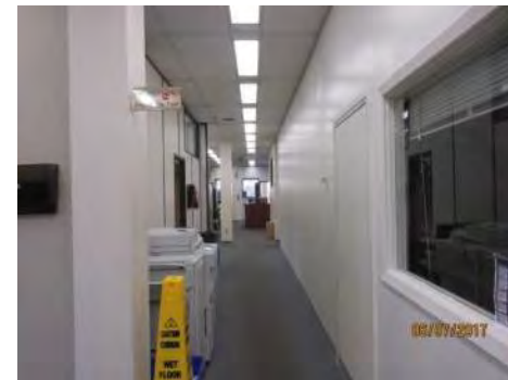
B42 2nd floor corridor: Corridor is well maintained. Clear width is suitable.
