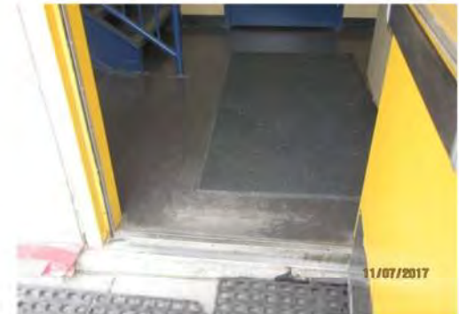
B3 Main entrance (north side): Transition is too high and entrance is not accessible. Clear door width is too narrow but suitable for an existing condition. Threshold ramp is in significant disrepair.
