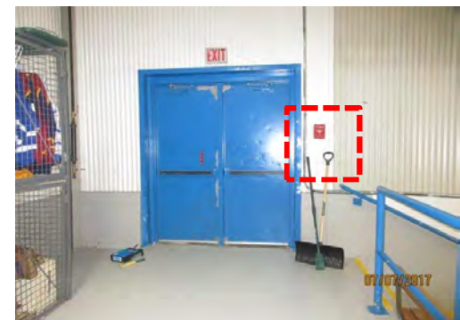
C6 Fire alarm pull, Upper Level, Viewing Stands (south side exit): Mounted too high for users of mobility aids.
