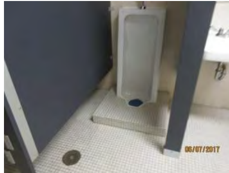
B110 2nd Floor, Men's Accessible Washroom (Staff): Urinal is not accessible due to step.
