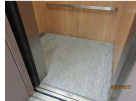
B51 Elevator: View of interior cab floor space. Handrail is provided on one side only.
