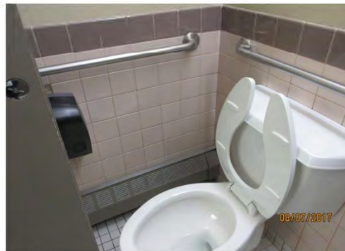
B65 Men's Accessible Washroom: Stall has limited clear floor space
