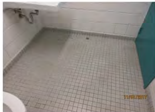
B22 Unisex Accessible washroom: Door swings inwards, which limits maneuverability when entering / exiting. Limited interior floor space, including area in front of lavatory, which generally allows side approach only.
