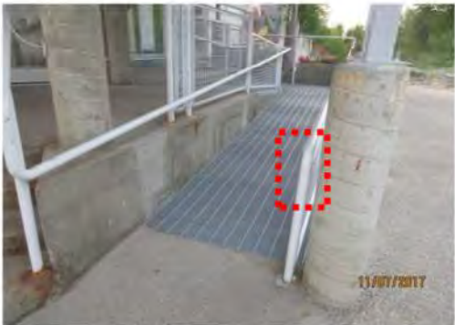
A28 Ramp adjacent to main entrance. Handrail extension is not provided on one side.
