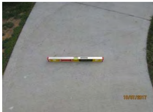
D70 Somba K'e Service Building (exterior): Cross-slope is too steep at some sections, exceeding 2%.
