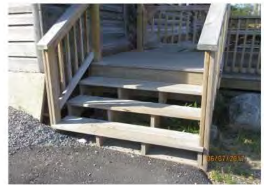
A12 Stair access only is provided to exterior deck. Open risers are potential tripping hazard. Handrails are oversized and difficult to grasp. Tread nosings are not high contrast.
