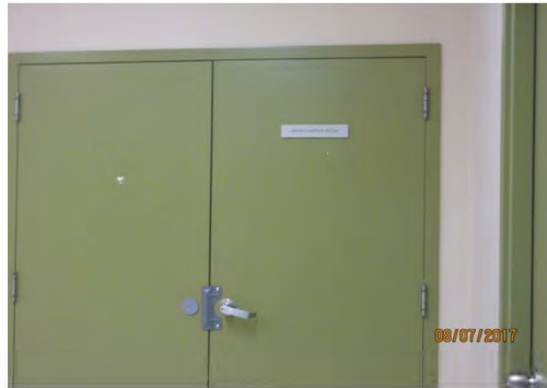
C13 Meeting Room: Identification signage text is too small. No accessibility features identified (e.g., tactile / braille).
