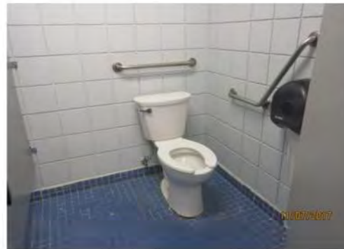
D20 Men's Change Room: Transfer space at side of toilet is too narrow. Stall dimensions and clear floor space is limited. Angled side grab bar is not preferred. Toilet paper dispenser is mounted too high and too far for reach.
