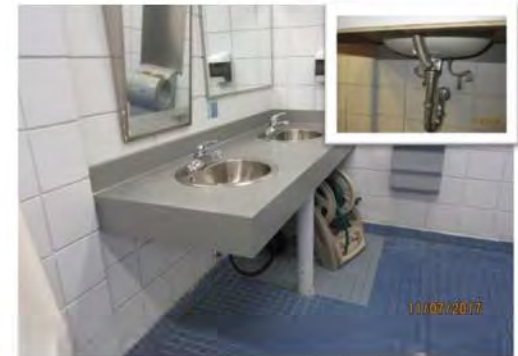
D21 Men's Change Room: Top surface height is suitable, however, knee space below is obstructed due to pipes. No pipe protection below lavatory. Angled mirror and lever faucet control are suitable.
