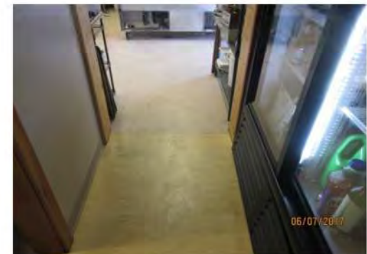
B18 Staff work area. Corridor to kitchen and exterior patio. Clear width is non-compliant and space is very constrained overall.
