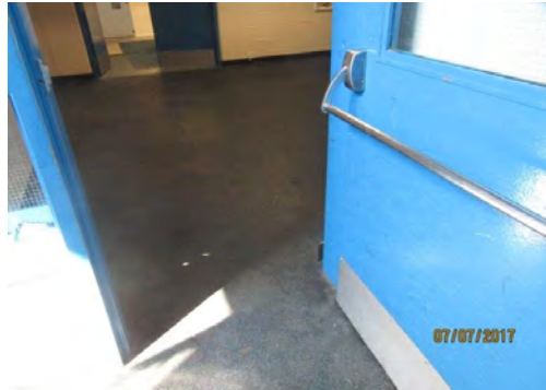
D19 Entrance to Lower Level, off of main stair: Typical clear width provided.
