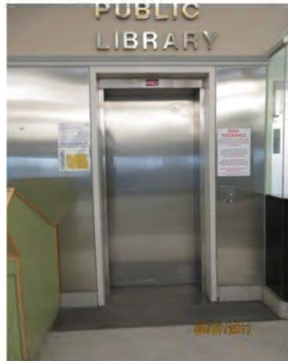
B13 View of Elevator lobby, off of mall, ground floor. Stainless steel surface, when highly polished, reflects glare which is a potential problem for users with vision loss.
