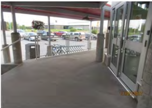
A20 Top landing area of stair and ramp at main entrance. No tactile warning surface indicator is provided at top of stair landing.
