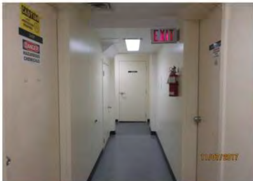
B28 1st floor, corridor to Dormitory (north west side): Where support columns project, some floor space is limited with no clear turning space for users of mobility aids (e.g., adj. to entrance to dormitory).
