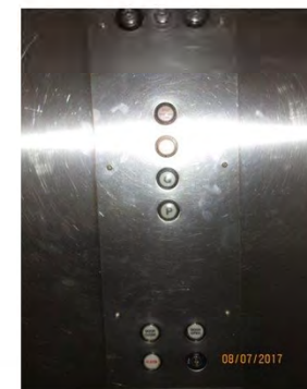
B48 Elevator cab control panel: No braille / tactile signage provided. Some buttons are mounted too high for users of wheeled mobility aids.
