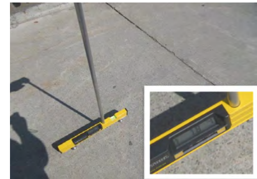
A12 Concrete surface, adjacent to main entrance: Excessive running-slope at 7.8% (adjacent to wall on north side of walkway).
