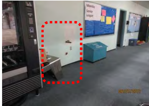
C7 Lower Level: Drinking fountain was not in working order and was not wall-mounted. Vending machine controls are not accessible.
