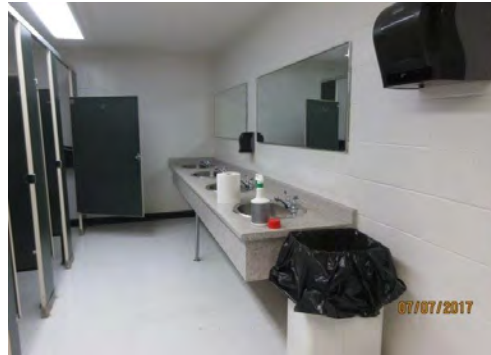
B32 Men's Accessible Washroom (Upper Level): No accessible lavatory is provided with knee space clearance below.
