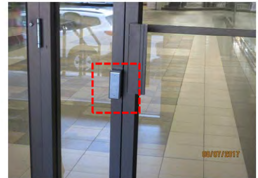
B6 Entrance (stair & ramp, 49th St.), interior side: Accessible entrance is not marked with ISA decal. A power door operator is provided, however, controls are too small and ISA symbol has faded. Adjacent door swings toward user and power door operator control and is potential bumping hazard.
