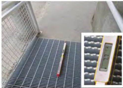
A27 Ramp, bottom section : Running slope is suitable at entry point, at 7.7%.
