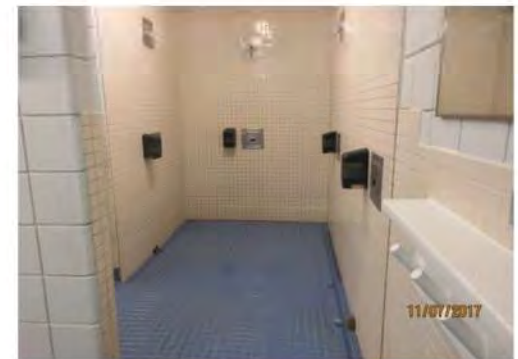
D24 Men's Change Room: Level access is provided into shower, however, no accessible features / controls were identified. Floor space is limited recognizing showers are multiple occupancy.
