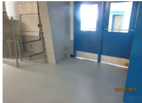
D17 Entrance to Enclosed Viewing Area from Ice Rink (Upper Level): No power door operator is provided. Lower edge of glazing is mounted too high.
