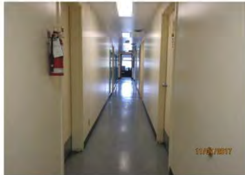
C4 1st floor: Typical wall-mounted fire extinguisher.
