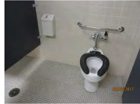
B99 Women's Accessible Washroom, main floor: Interior features are non-compliant.
