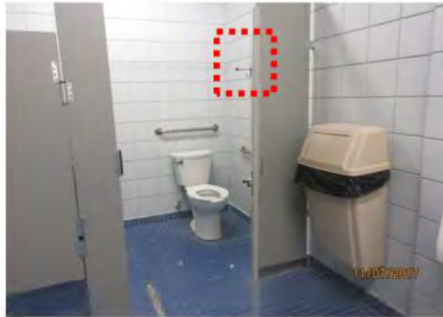
D19 Men's Change Room: Entrance door is not self-closing. Coat hook is mounted too high.
