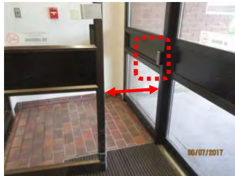
B4 Clearance between doors is non-compliant and very limited. Use of PDO control for exterior door is obstructed by door swing.
