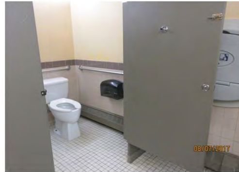
B74 Women's Accessible Washroom: Stall has limited clear floor space. Stall door is not self closing and coat hook is too high. Door clear width is too narrow.
