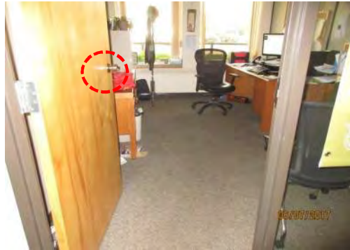
D37 Private Office, Main Floor (south side): Door clear width is suitable for existing condition. Knob door hardware is not accessible.
