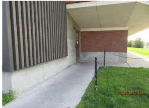
A14 Approach to rear staff entrance / exit (north east side of site). No problems were identified. Chains mounted between posts are not cane detectable for users with vision loss and may result in potential bumping / tripping hazards.
