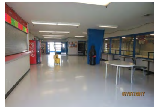
B12 Enclosed Viewing Area and Concession Stand (looking south): No accessible or lowered counter is provided at Concession window.
