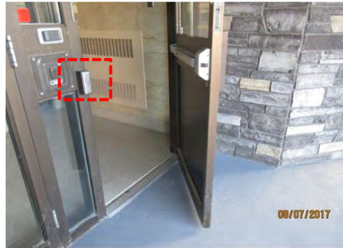
B2 Entrance (stair & ramp, 49th St.): A power door operator is provided, however, controls are too small. Door swings towards user and top landing area of ramp.
