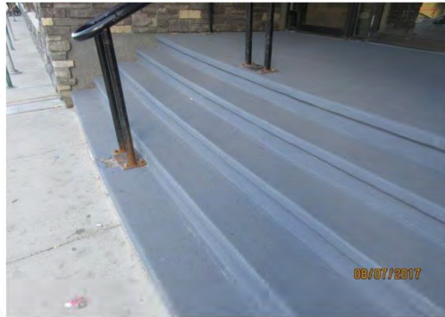
A19 Stairs: No colour contrasted nosings are provided. A centre handrail is provided only. No handrails are provided on other sides of stairs.
