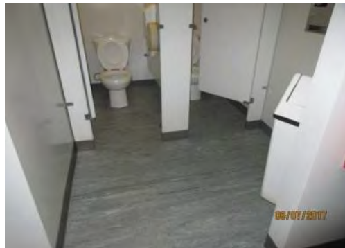
B46 Main Floor (adj. to secondary entrance): Women's Washroom. Identified as accessible through door signage but it is not accessible.
