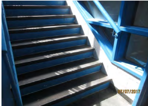
B19 Central Stair: Handrail grasping dimension is too large. No handrail extensions are provided at bottom landing.
