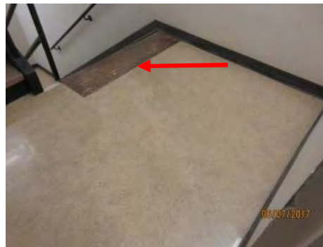
B80 Stair #1 (northeast side, 2nd floor): No TWSI is provided at top landings.
