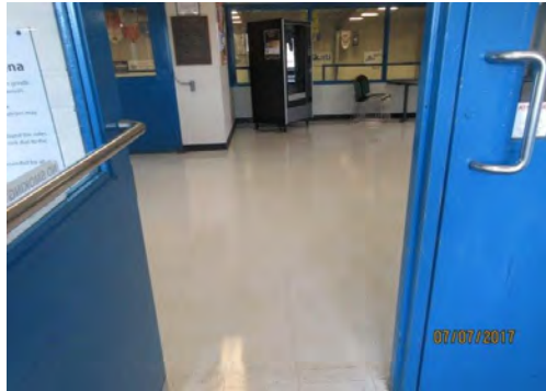
B7 Main accessible entrance vestibule: Interior door is not marked with the International Symbol of Accessibility (ISA) decal. Clear door width is non-compliant (too narrow).
