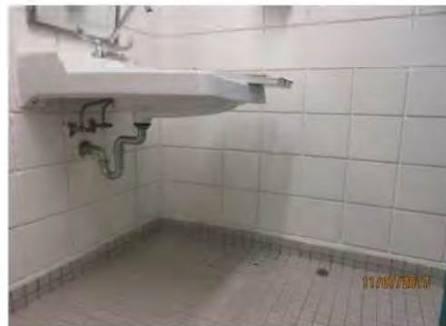
B23 Unisex Accessible washroom: Some interior amenities are non-compliant and overall, maneuverability is problematic due to limited interior floor space, including area in front of lavatory.
