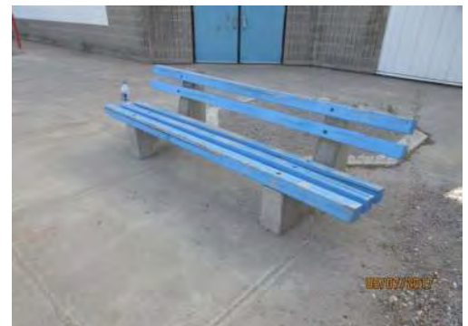
A12 Bench is not accessible and is dated construction.
