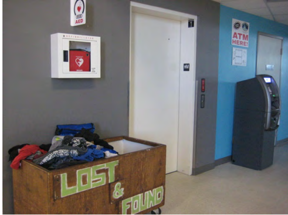
C1 AED cabinet in main lobby to the left of elevator.
