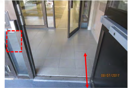
B3 Entrance (stair & ramp, 49th St.): Exterior door glazing is mounted too high.
