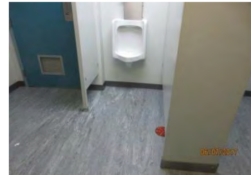
B36 Main Floor (adj. to entrance): Men's Washroom. Identified as accessible through door signage but it is not accessible.
