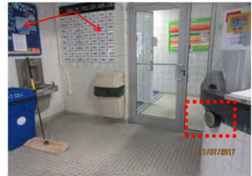
B6 View of entrance to Pool Change Rooms: Power door operator is provided. Door is not marked with international symbol of accessibility decal. Generally, information on display is posted too high.
