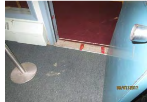
D9 Entrance, Curling Rink (accessed from Lower Level): Level access at entry #1 and suitable clear door width is provided for an existing condition, however, no elevator access is provided to this level.
