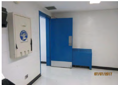
B28 Men's Accessible Washroom (Upper Level): Entrance doors have limited clear width but typically suitable for an existing condition. No power door operator is provided.
