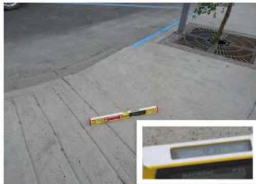
A10 Curb ramp (south east side, adj. to on-street accessible parking space): Running slope of flared side is suitable at 9%.
