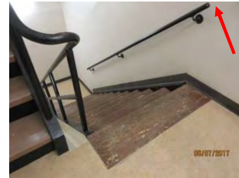
B81 Stair #1 (northeast side, 2nd floor): Stair treads do not have colour contrasted nosings. No handrail extensions are provided.
