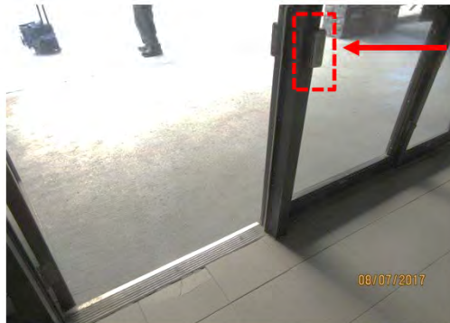
B16 Entrance (Sloped route), exterior vestibule door: Level access is provided and threshold is suitable. Power door operator control is too small.
