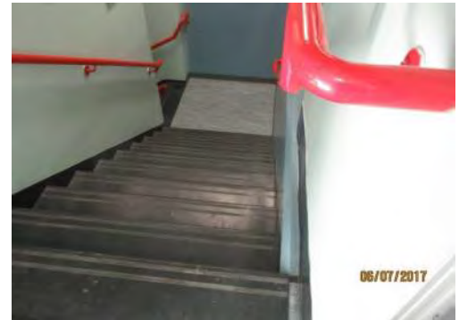
B30 Stair #2: No TWSI provided at top landing. No colour contrast is provided on stair tread nosings for users with a vision loss. Handrails have large grasping surface / dimension.
