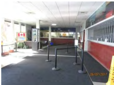
B22 2nd floor, entrance lobby: Line up guides do not have cane detectable lower edge which may result in bumping / tripping hazard for users with a vision loss.
