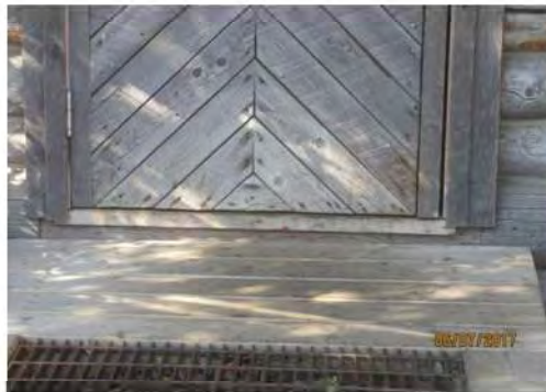
B4 Main entrance: High threshold and openings for grating are not accessible.
