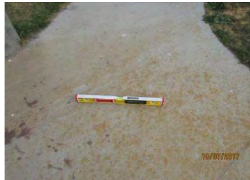
D76 Somba K'e Service Building (exterior): At lower section of walkway, cross-slope is suitable at 2% or less.
