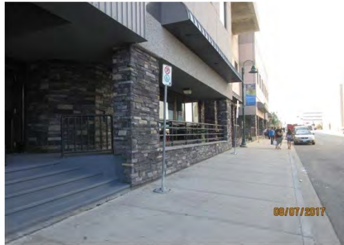
A1 Approach to Library entrances, off of 49th Street and adjacent to stair / ramp entrance. Post-mounted signage is provided to designate on-street accessible parking. No pavement markings, access aisle or curb ramp identified for accessible parking.
