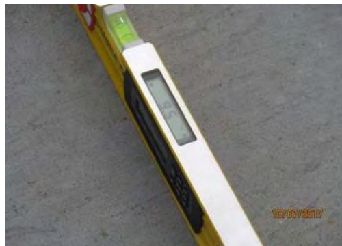
D69 Somba K'e Service Building (exterior): Running slope of walkway to entrance (upper section) is too steep in multiple sections, for users of mobility aids, exceeding 9%.
