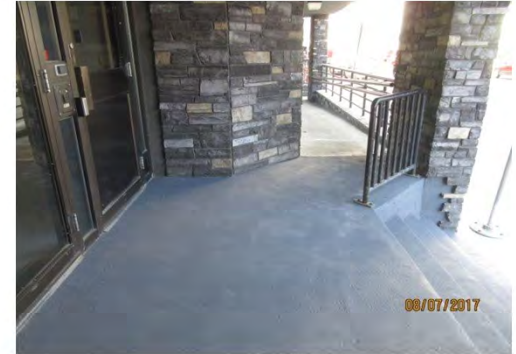
A15 View of top landing of stair and ramp. Landing is awkward configuration by door. Power door swings towards top landing of ramp which is a potential bumping hazard. No TWSI is provided at top of stair landing.
