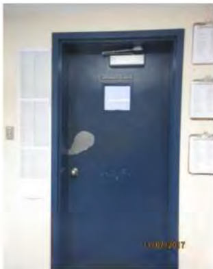
B26 1st floor, entrance to Apparatus / Truck Bays: Clear door width and hardware is non-compliant.
