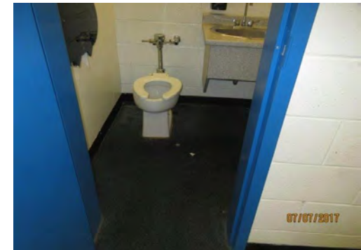
D30 Referee's / Official's Change Room (Lower Level, north side): Entry clear width is too narrow. Interior dimensions limited.
