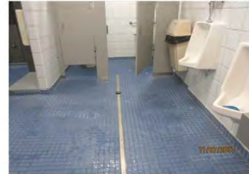
D18 Men's Change Room: View of clear floor space adjacent to urinals and approach to accessible stall. Cross-slope of some areas of floor surface is non-compliant and designed for drainage.
