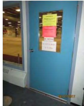
D8 Curling Rink (accessed from Lower Level): Level access at entry #1 and suitable clear door width is provided for an existing condition, however, no elevator access is provided to this level.
