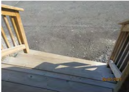
A13 Stepped access only is provided to exterior deck. No colour contrasted nosings are provided. Handrail is oversized.
