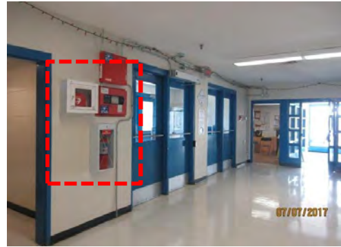
C5 Upper Level, Enclosed Viewing Area & Entrance Lobby: Safety equipment typically mounted too high for users of mobility aids.
