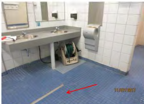
D22 Men's Change Room: Clear floor space in front of lavatory is uneven.
