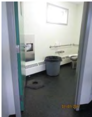
D94 Somba K'e Service Building (interior): Men's washroom is not accessible. Clear door width is limited but suitable for existing condition. Lever door hardware is provided. No power door operator is provided.
