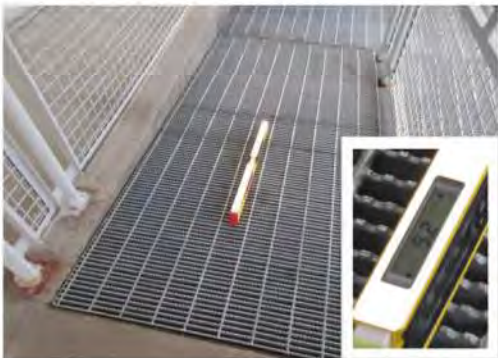
A23 Ramp, top section (adj. to entrance): Running slope is too steep and non-compliant at 9.2%.
