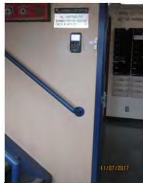
B5 Main entrance vestibule: Typical information / directional signage and operating controls are not accessible.
