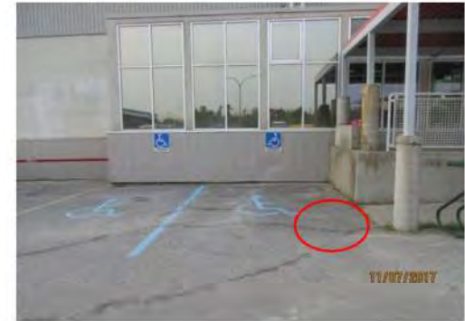
A9 Accessible spaces are marked with pavement and wall-mounted signage. No access aisle is provided between two spaces and to prevent vehicle from blocking accessible route to main entrance when vehicle is parked (red circle area).
