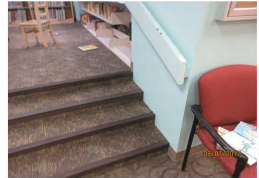
B39 Kids Area: Colour contrast of stair nosings is limited. Handrails are not accessible. No TWSI is provided at top landing. Raised platform is not accessible for users of wheeled mobility aids.
