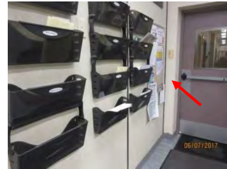
B75 Entrance to Stair #1 (interior door, northeast side): Clear door width is suitable for existing condition. Bottom edge of door glazing is mounted too high. Required clear wall space at latch side of door is not provided. (Note: Level access to exterior is not provided at this exit stair due to high transition)
