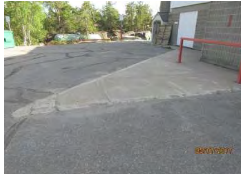
A8 No curb ramp is provided. Transition between parking area and sidewalk leading to secondary entrance is too high for users of mobility aids.
