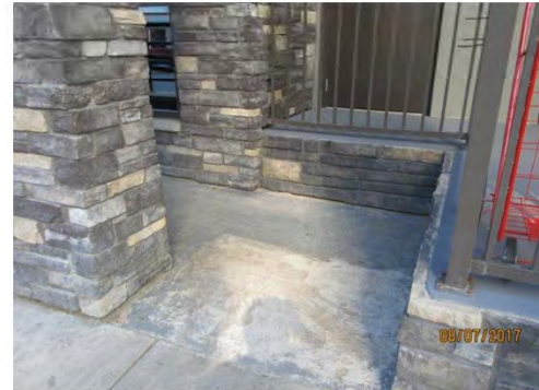
A5 Ramp entry (bottom landing): Surface is in disrepair. Clear width is too narrow and landing size is too small.
