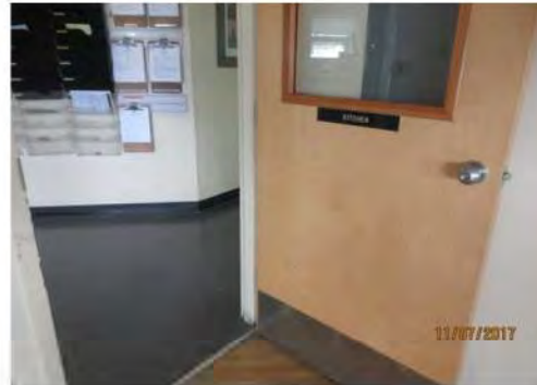
D8 1st floor, Kitchen entrance #1: Clear door width is suitable for an existing condition. Knob door hardware is not accessible. Lower edge of vision panel is too high.
