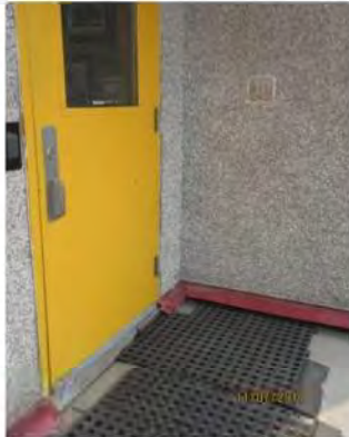
B1 Main entrance (north side): Not accessible due to step, door clear width, glazing and hardware design.
