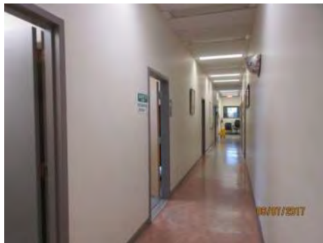
B40 2nd floor, approach to Staff Kitchen and Lunchroom: Corridor is well maintained.
