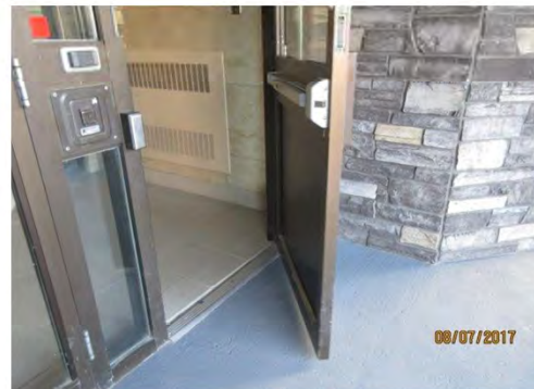
A17 View of top landing of stair and ramp. Landing depth is very limited. Power door swings towards top landing of ramp which is a potential bumping hazard.
