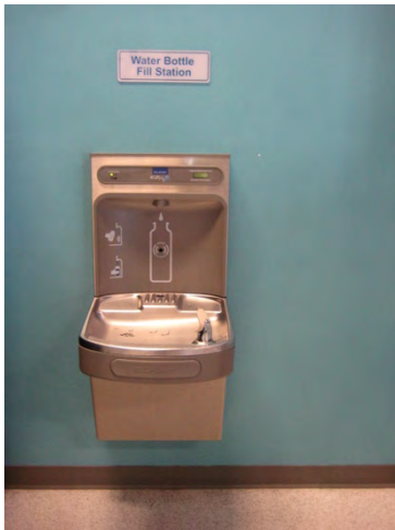
C3 water fill in main lobby area
