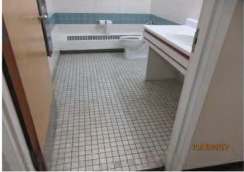
B33 2nd floor, entrance to Washroom #1: Clear width is suitable. No accessibility features identified. However, 2nd floor is not accessible.
