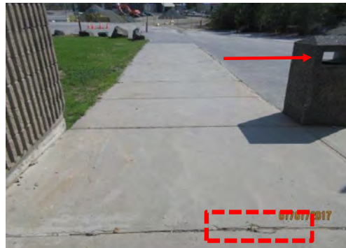
A8 Approach to main entrance (west side). Some heaving / settlement between concrete sections observed. No seating/rest areas identified, with limited to no amenities / street furniture. One accessible waste receptacle identified adjacent to main entrance.
