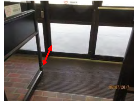
B6 Clearance between doors is non-compliant and very limited. Use of PDO control for exterior door is obstructed by other door swinging towards control.
