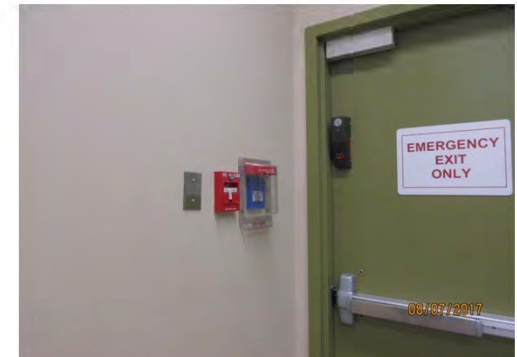
B78 Exit Stair (adj. to Meeting Room): Fire alarm pull is mounted too high. Appeared to be typical condition throughout.
