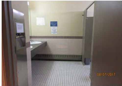
B61 Men's Accessible Washroom: Limited interior clear floor space, especially for users of larger wheeled mobility aids.
