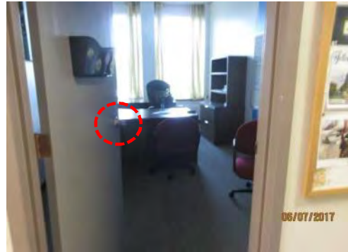
D44 Private Office, 2nd floor (east side). Typical entrances have limited clear width and knob door hardware which is not accessible.
