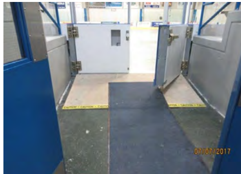
D23 Sloped corridor and temporary ramping leading to Gate #1 (Central) to Ice Surface: Ramping is non-compliant.
