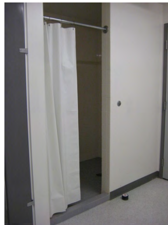
D18 shower stall in washrooms connected to soccer field change rooms (typical)
