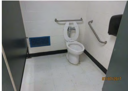
B31 Men's Accessible Washroom (Upper Level): Stall floor space is limited. Flush control is mounted on transfer side of toilet. Stall doors are not self closing. No L-shaped grab bar is provided at side of toilet. Toilet paper dispenser mounted too far and too high.
