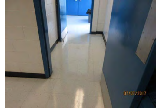
B27 Men's Accessible Washroom (Upper Level): Entrance doors have limited clear width but typically suitable for an existing condition.
