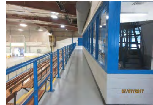
D12 Corridor (Upper Level, north side): Suitable clear width is provided, although it is limited to allow one way traffic only.
