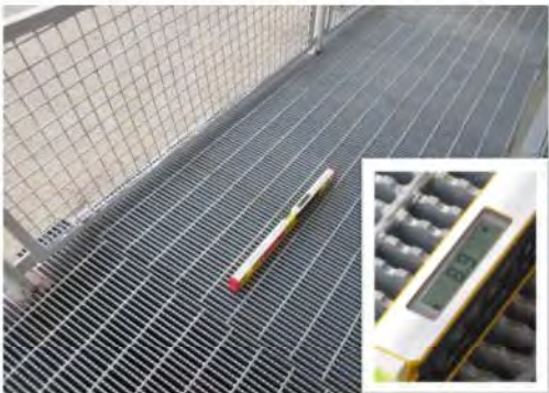
A25 Ramp: Running slope is too steep at 8.9%, for section at lower end of ramp.
