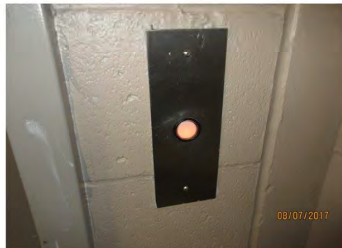
B53 Elevator lobby, parking garage: Hall call buttons are illuminated when activated.
