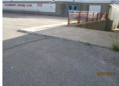
A14 No curb ramp is provided. Transition between parking area and sidewalk leading to main entrance is too high for users of mobility aids.
