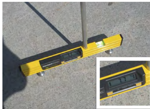
A11 Concrete surface, adjacent to main entrance: Excessive running-slope at 7.8% (adjacent to wall on north side of walkway).
