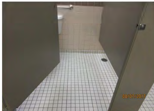
B64 Men's Accessible Washroom: Stall has limited clear floor space. Door clear width is too narrow.
