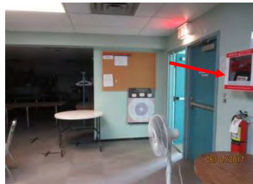
C5 AED Cabinet: Bottom edge is not cane detectable for users with a vision loss, therefore projection from wall is a potential bumping hazard for users with a vision loss.
