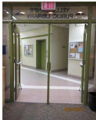
B22 Main entrance, Library, 2nd floor. Door clear width is not compliant. Doors appear to be kept propped open during regular operating hours.
